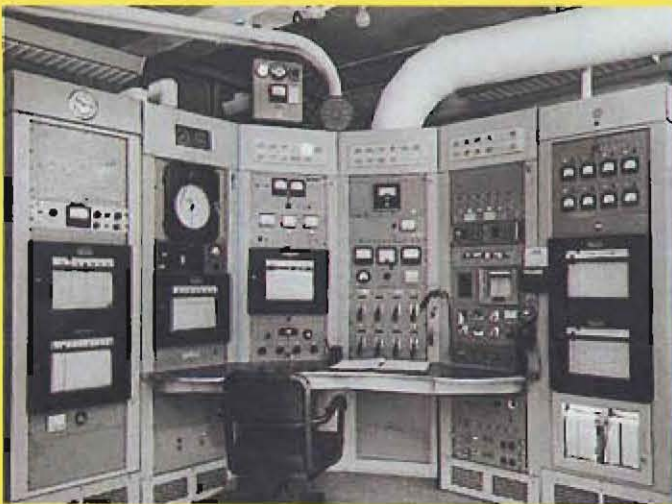
OWR Control Panel
