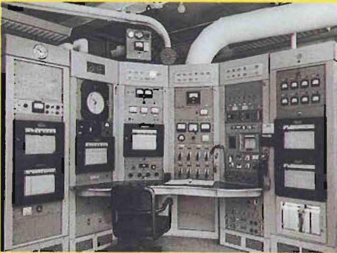
OWR Control Panel
