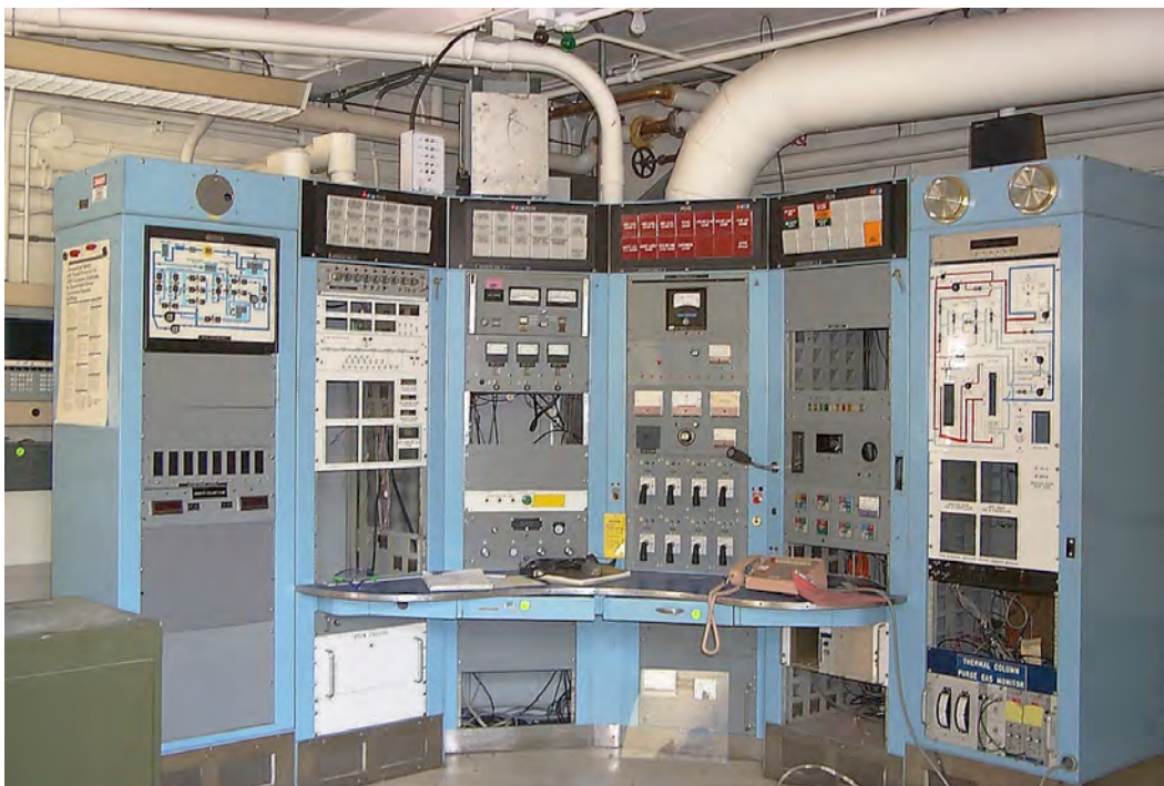
Figure 14.5. Omega West Reactor Control Panel at TA-2.
