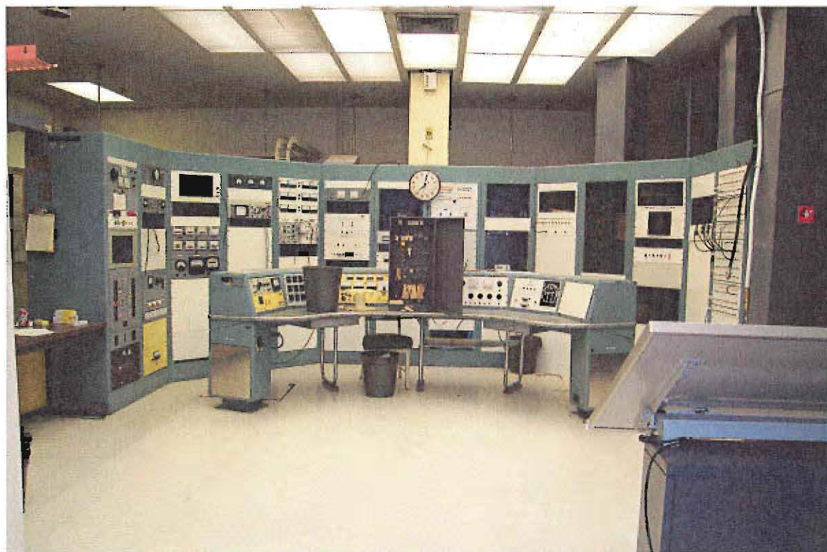
Figure 4. Van de Graaff Accelerator Control Room
