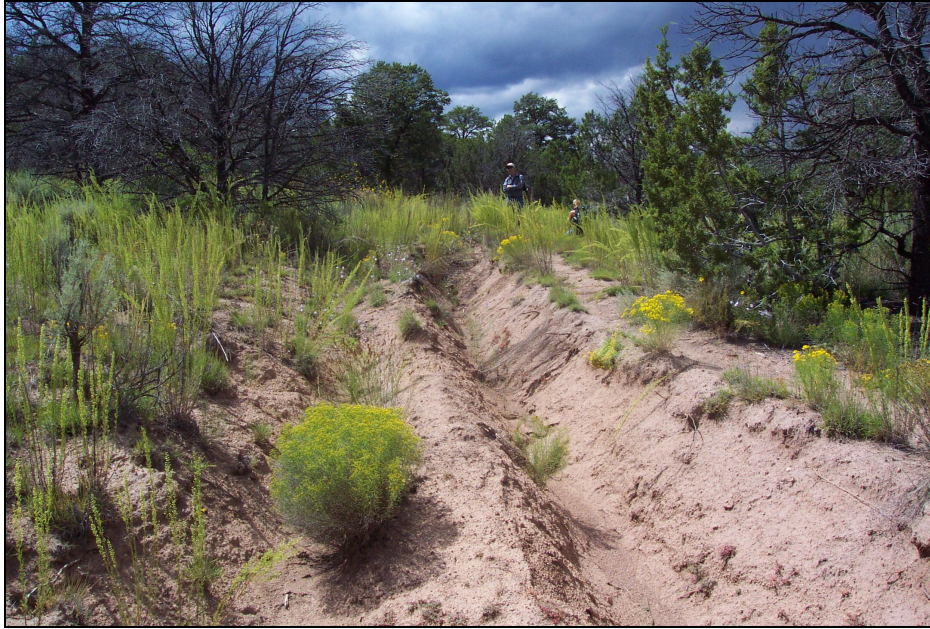
Figure 9. Heavily eroded trail segment 4-E.
