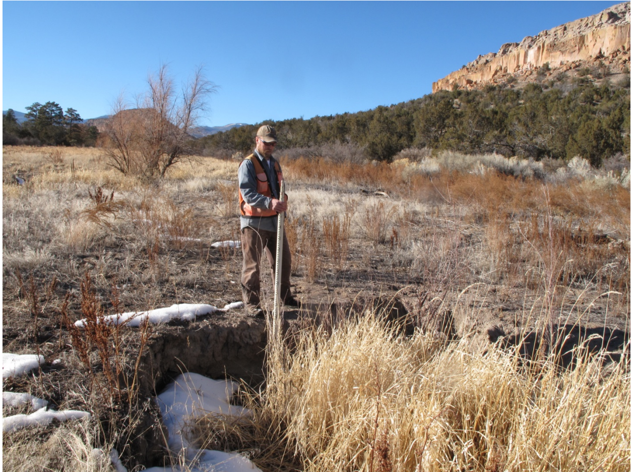
Photo A1-8 January 2013 photograph of southern headcut at cross-section PU 0 ft, in the lower half of the lower Pueblo Canyon willow-planting area, where the emergence of alluvial groundwater perched on Puye Formation bedrock results in seepage erosion. Wetland vegetation and willows are established below headcut.
