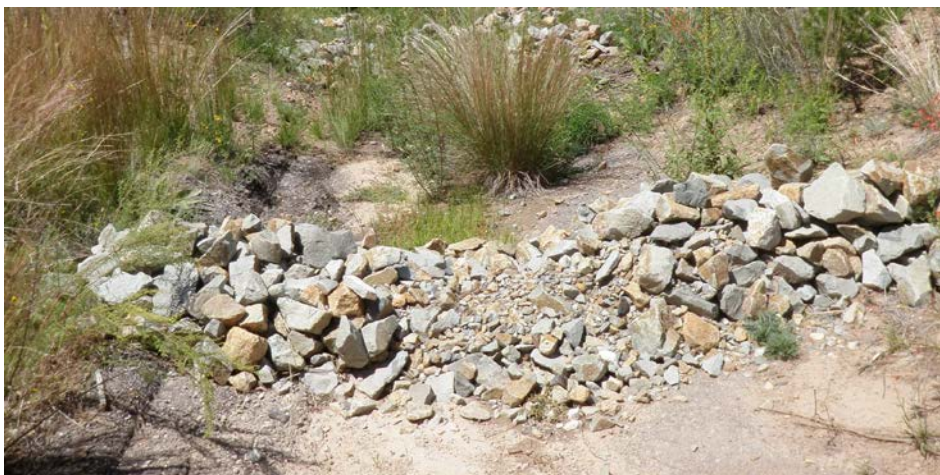
S-SMA-3.71, Rock Check Dam, S00806010008 (photo ID 8515-2)
