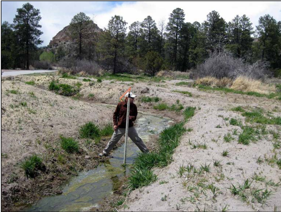
Photo A1-7 May 2014 photograph of area of maximum sediment erosion below the Pueblo Canyon wing ditch at cross-section WD-4, looking upstream
