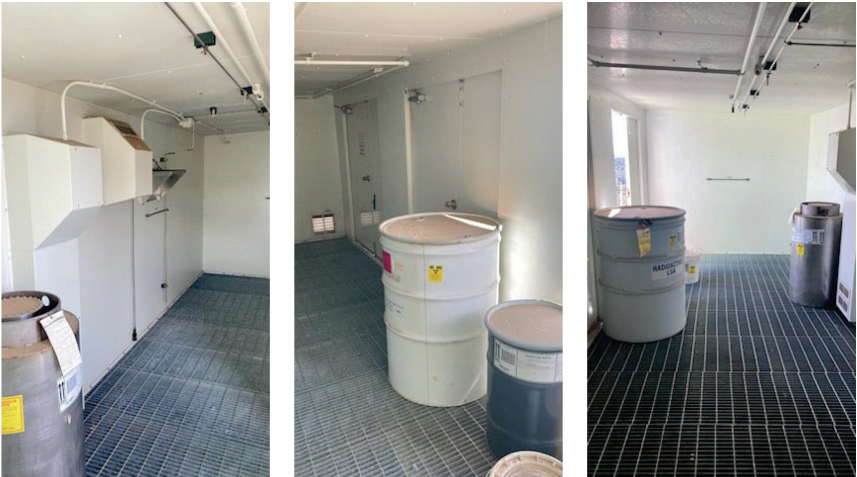
Figure 10: Inside TA-54, Area G, Pad 5, Building 1028 after FTWC and temporary equipment removal
