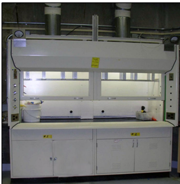
Figure 2.9-1. Example of a laboratory fume hood at LANL
