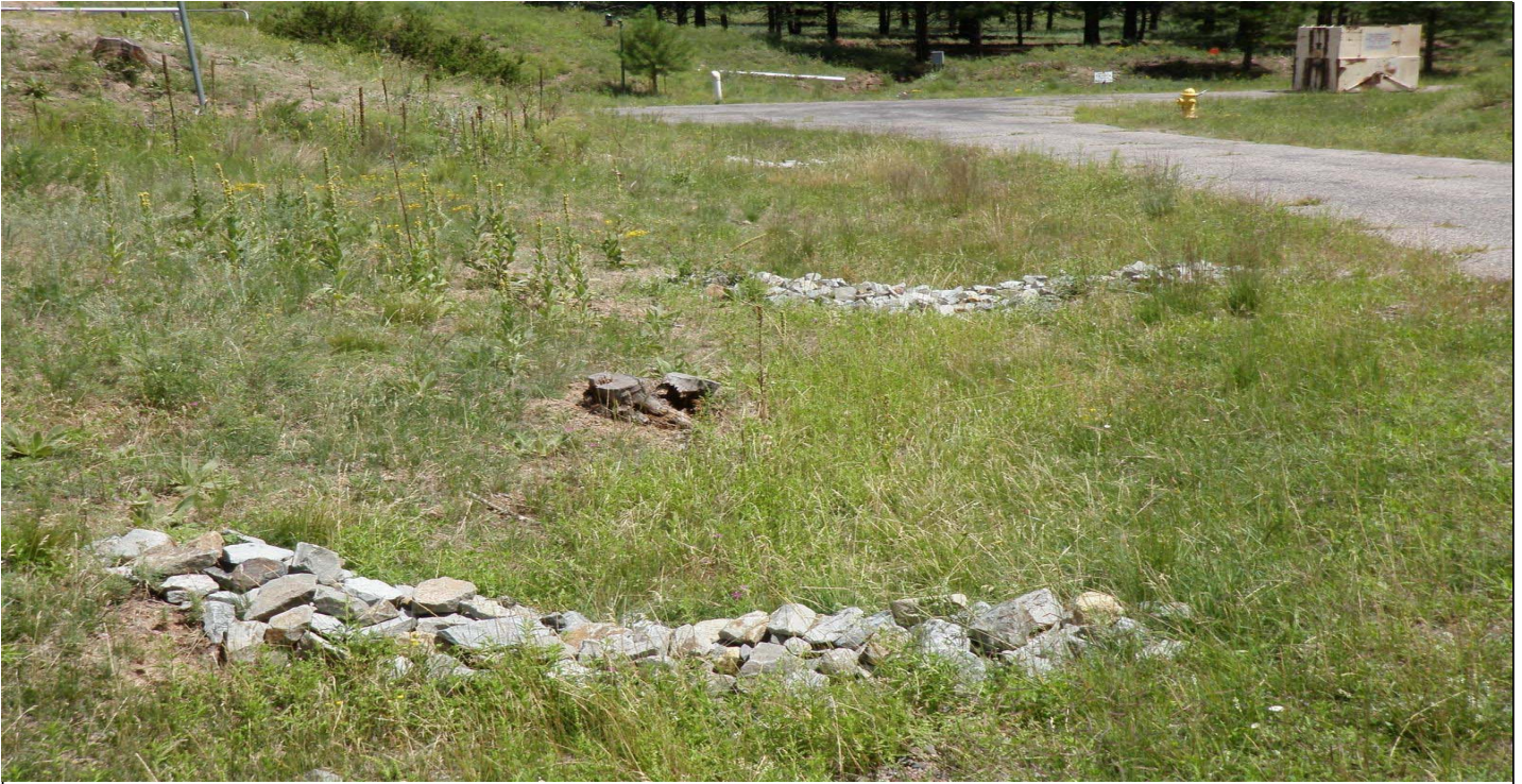
Photo 7594-1r.JPG (taken 08/13/10) W00106010008 : Check Dam - Rock Check Dam; W00106010009 : Check Dam - Rock Check Dam; W00106010010 : Check Dam - Rock Check Dam.
