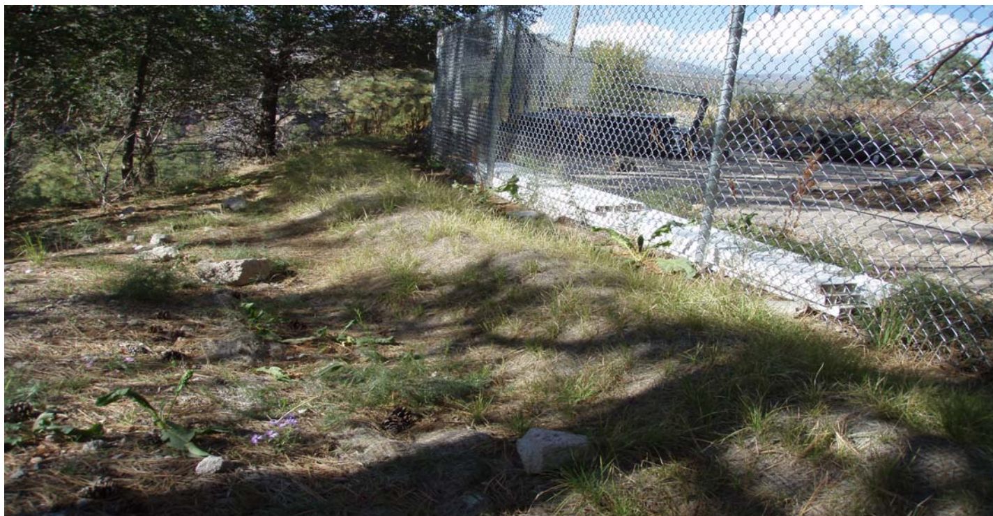
Photo 10871-9.JPG (taken 10/07/10) P00301060010 : Seed and Mulch - Erosion Control Blanket; P00303010009 : Berms - Earthen Berm.
