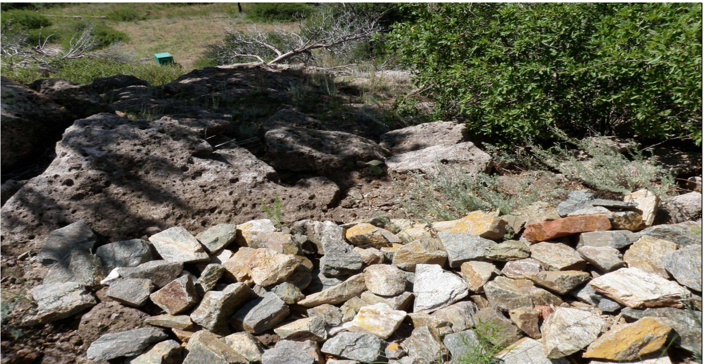
Photo 7486-4r.JPG (taken 08/10/10) M01606010007 : Check Dam - Rock Check Dam.
