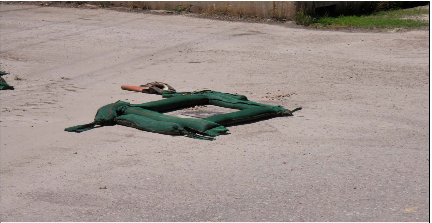
Photo 7427-2.JPG (taken 07/28/10) L01403100003 : Berms - Gravel Bags.
