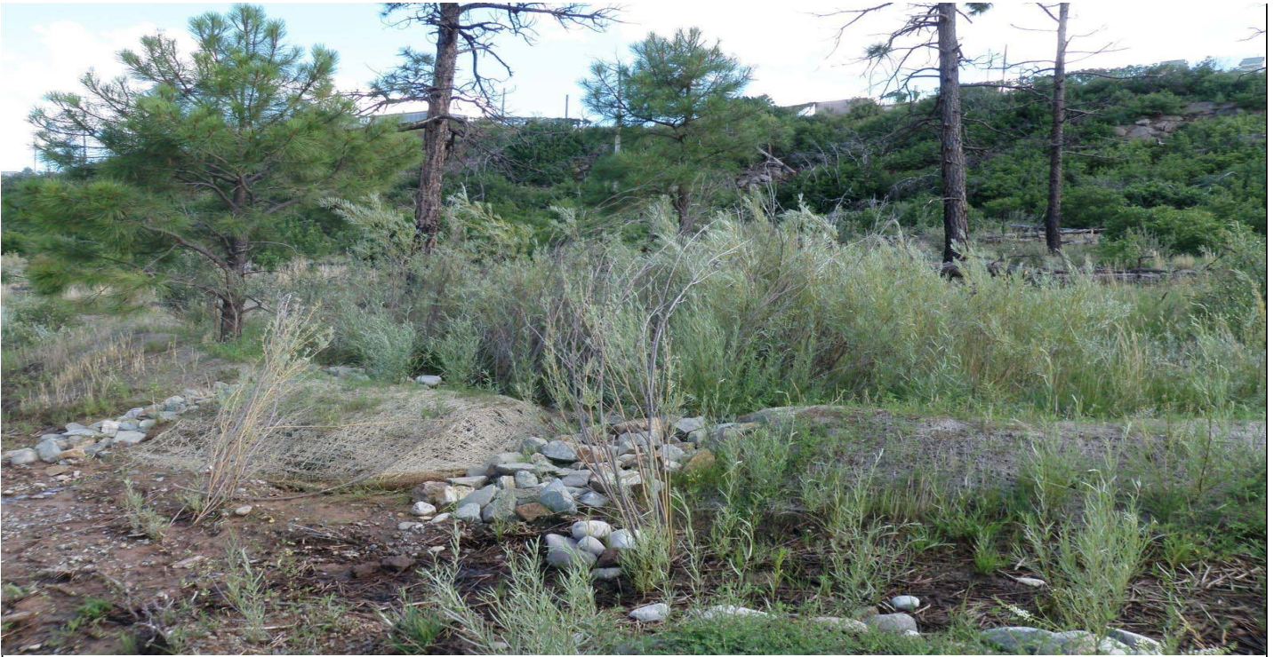
Photo 7484-1r.JPG (taken 08/10/10) C00201060014 : Seed and Mulch - Erosion Control Blanket; C00202010005 : Established Vegetation - Permanent Vegetation Grasses and Shrubs; C00203010013 : Berms - Earthen Berm.
