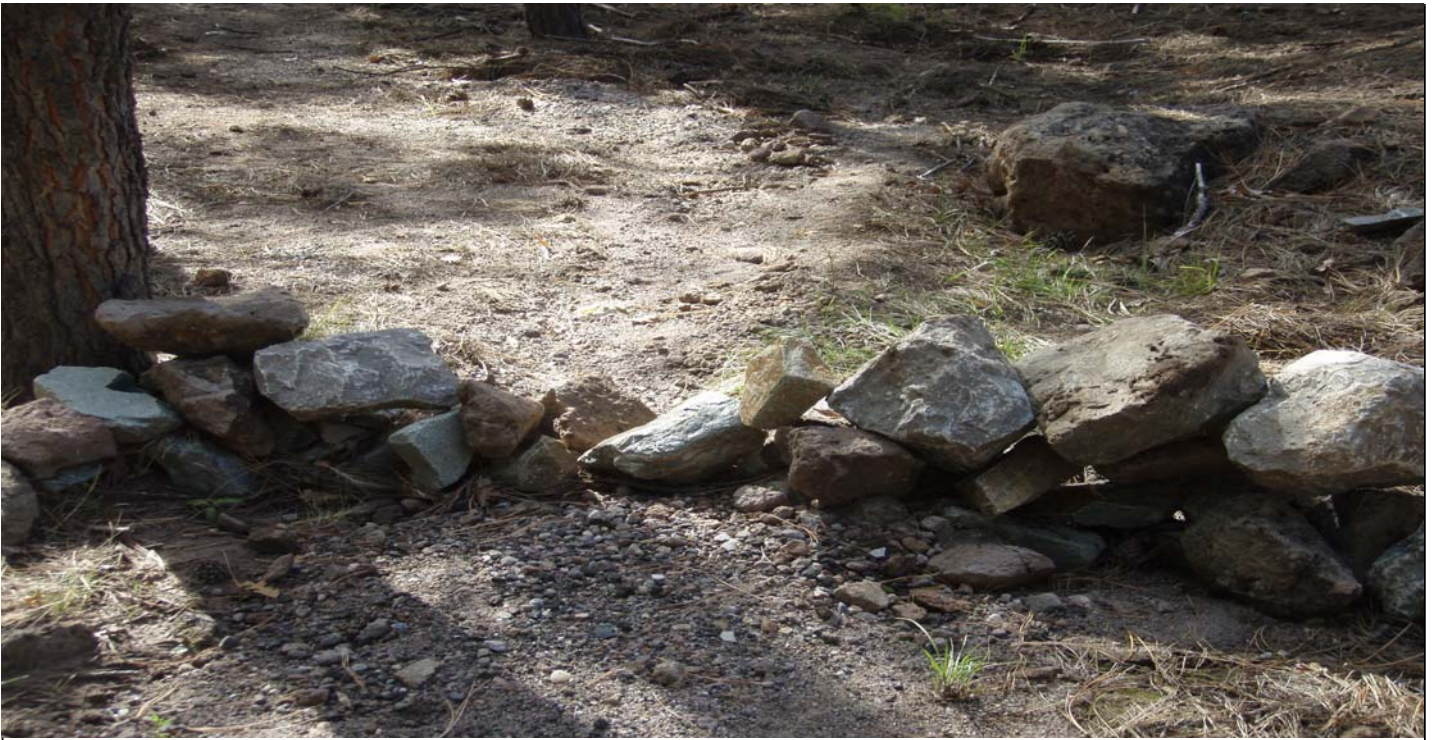
Photo 10870-1.JPG (taken 10/07/10) P00206010013 : Check Dam - Rock Check Dam.
