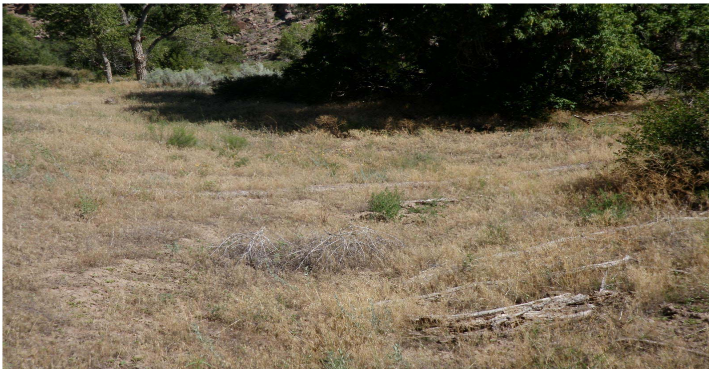
Photo 7528-2r.JPG (taken 08/12/10) J02303060002 : Berms - Straw Wattles.
