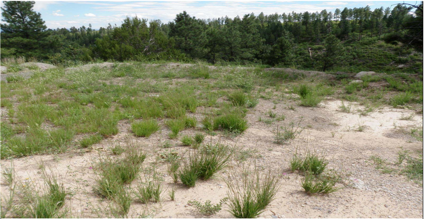
Photo 7510-3r.JPG (taken 08/12/10) J00901060007 : Seed and Mulch - Erosion Control Blanket; J00903010009 : Berms - Earthen Berm.
