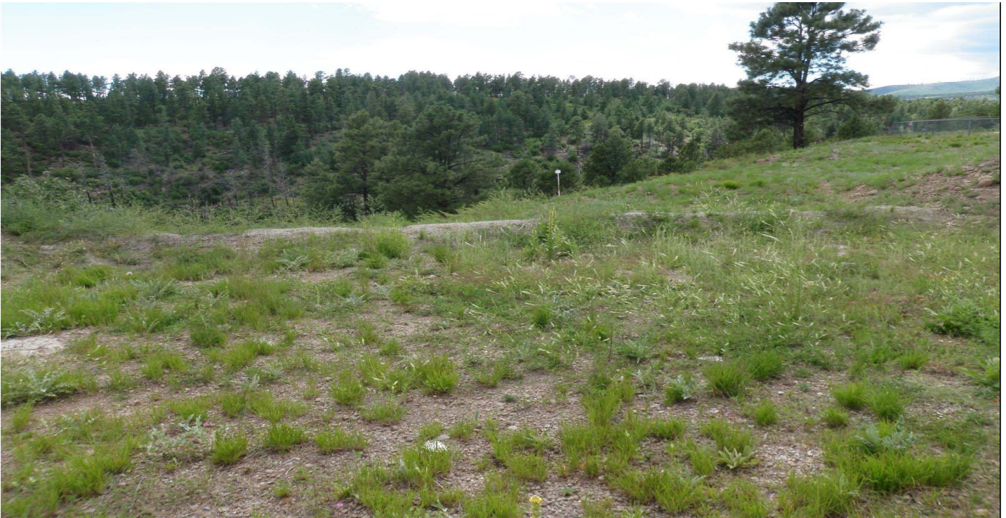
Photo 7510-2r.JPG (taken 08/12/10) J00901060008 : Seed and Mulch - Erosion Control Blanket; J00902010003 : Established Vegetation - Permanent Vegetation Grasses and Shrubs; J00903010006 : Berms - Earthen Berm.
