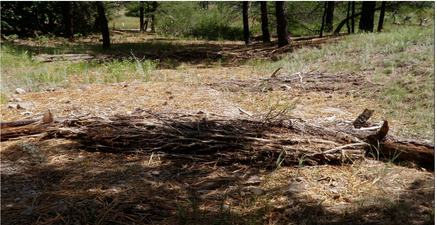
Photo 7414-3.JPG (taken 07/29/10) D00501010010 : Seed and Mulch - Seed and Wood Mulch; D00506030007 : Check Dam - Juniper Bales; D00506030008 : Check Dam - Juniper Bales.
