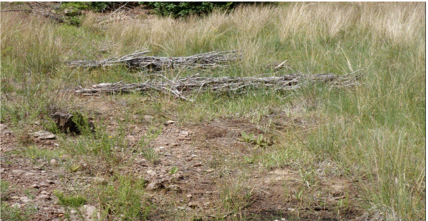
Photo 7506-6r.JPG (taken 08/11/10) J00502010006 : Established Vegetation - Permanent Vegetation Grasses and Shrubs; J00506030007 : Check Dam - Juniper Bales.
