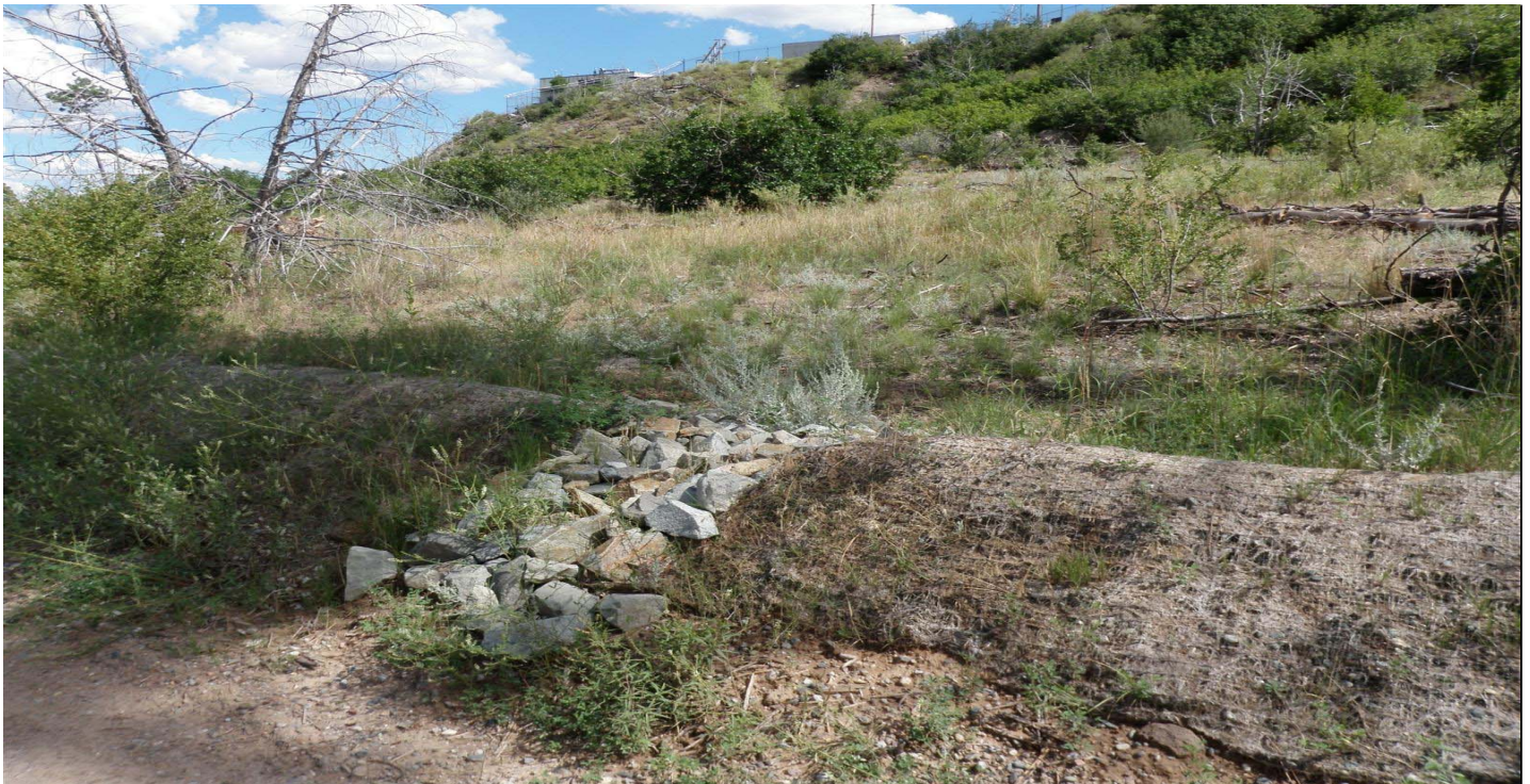
Photo 7483-1r.JPG (taken 08/10/10) C00501060009 : Seed and Mulch - Erosion Control Blanket; C00502010005 : Established Vegetation - Permanent Vegetation Grasses and Shrubs; C00503010006 : Berms - Earthen Berm.
