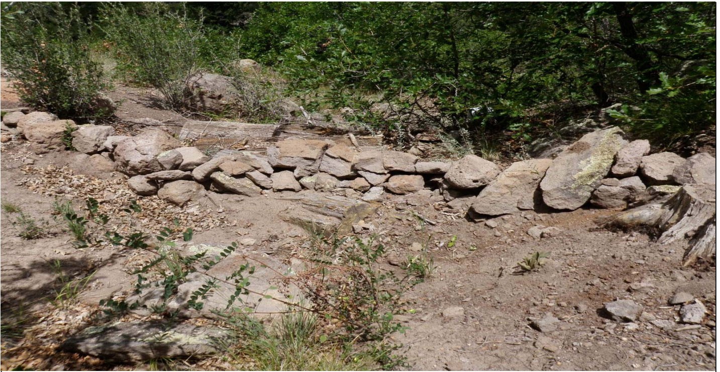
Photo 7417-1.JPG (taken 07/30/10) P00603120008 : Berms - Rock Berm.
