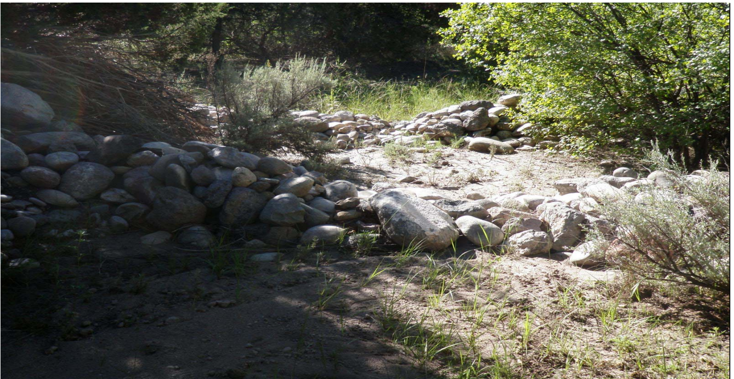
Photo 8505-6r.JPG (taken 08/20/10) J02506010007 : Check Dam - Rock Check Dam; J02506010008 : Check Dam - Rock Check Dam.
