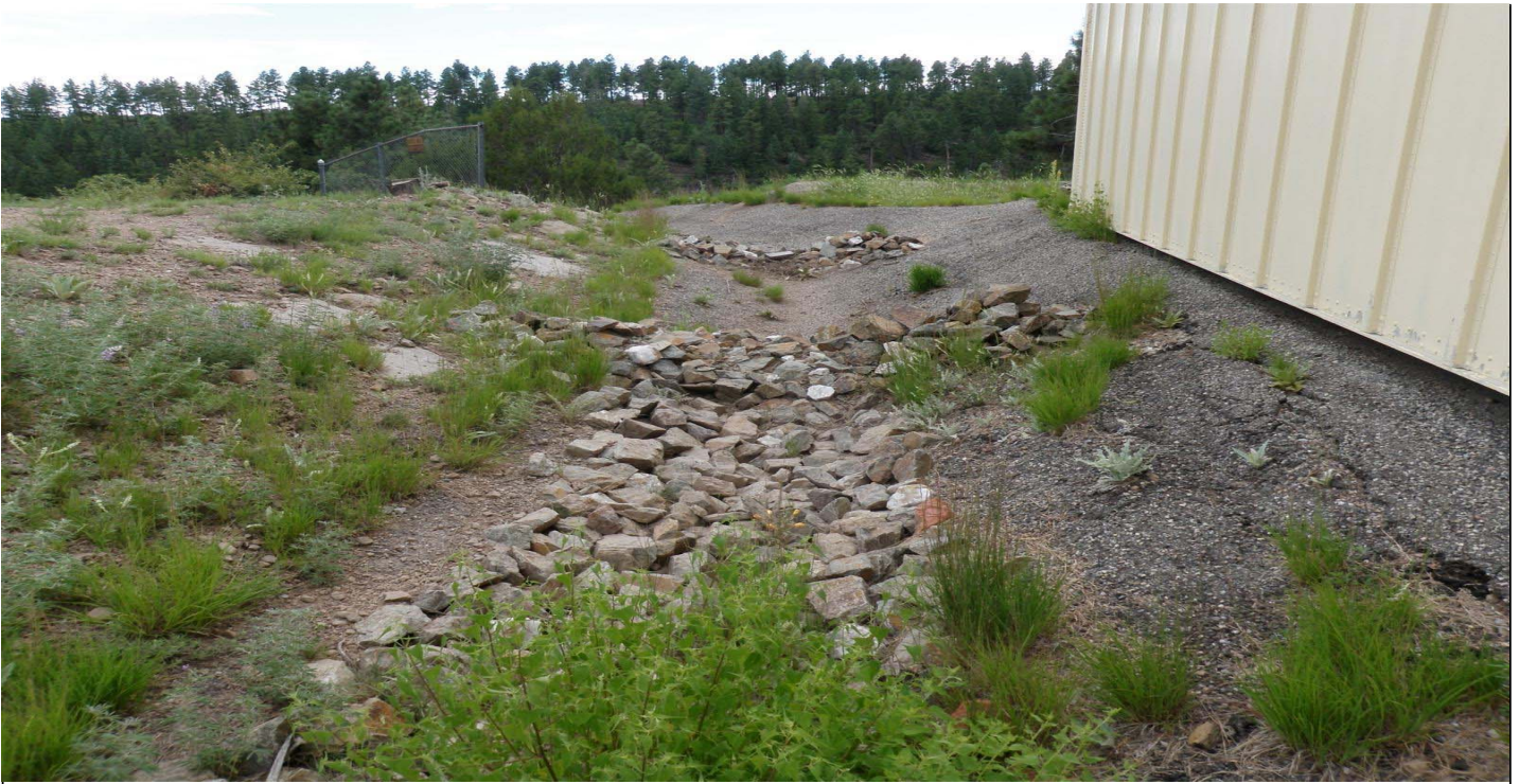
Photo 7510-1r.JPG (taken 08/12/10) J00904020005 : Channel/Swale - Concrete/Asphalt Channel/Swale; J00904060001 : Channel/Swale - Rip Rap; J00906010002 : Check Dam - Rock Check Dam; J00906010004 : Check Dam - Rock Check Dam.
