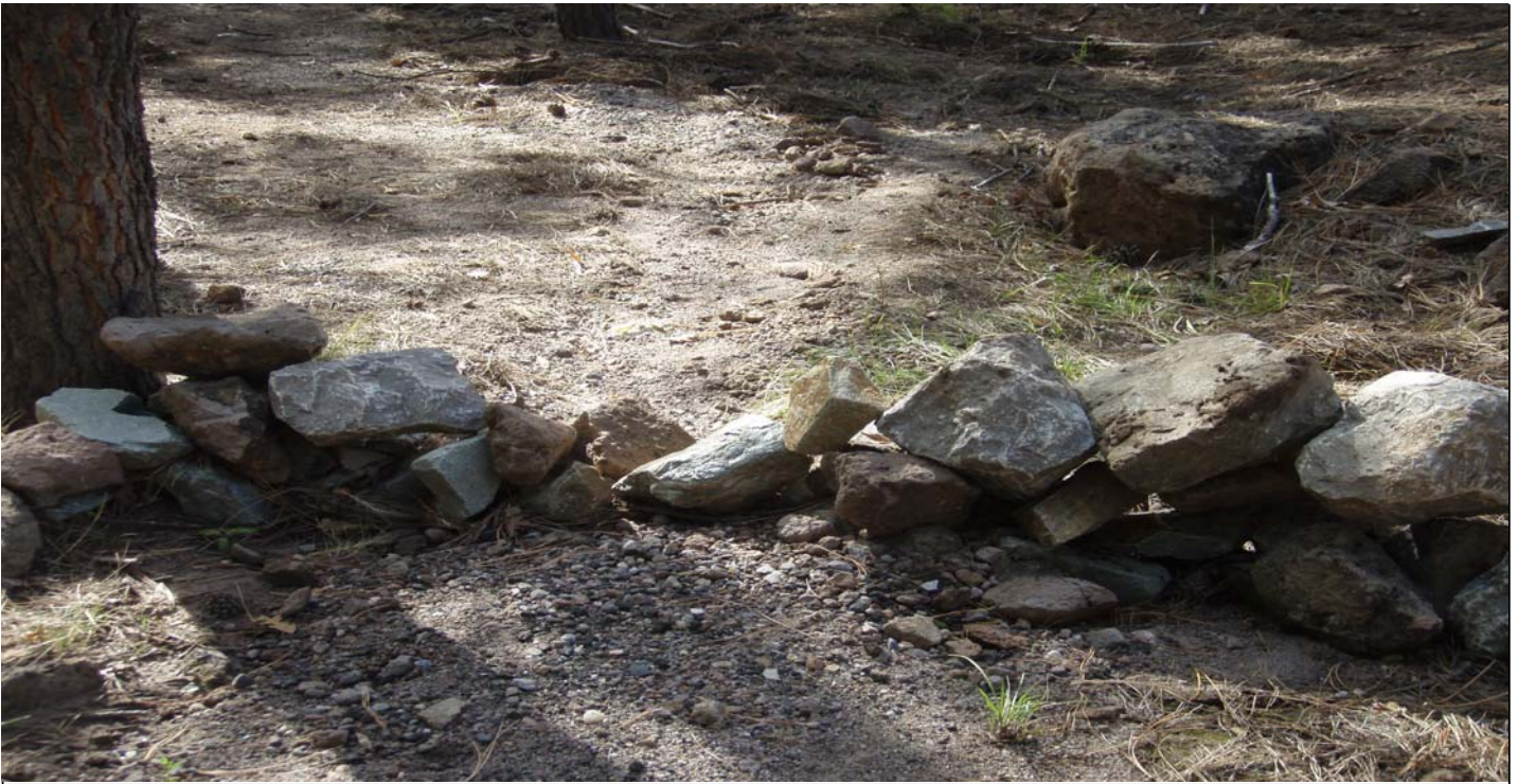
Photo 10871-2.JPG (taken 10/07/10) P00306010015 : Check Dam - Rock Check Dam.
