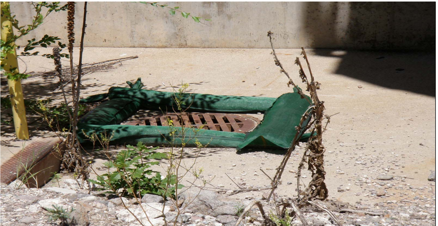
Photo 7427-3.JPG (taken 07/28/10) L01403100006 : Berms - Gravel Bags.
