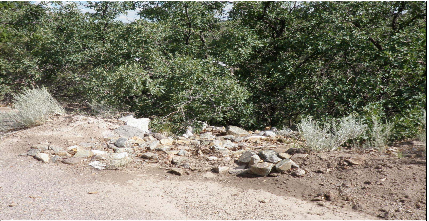
Photo 7480-1r.JPG (taken 08/09/10) M00606010005 : Check Dam - Rock Check Dam.
