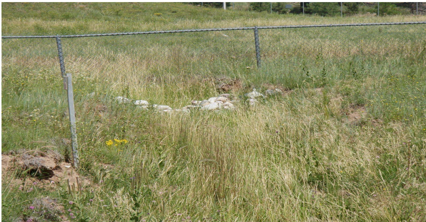
Photo 7504-2r.JPG (taken 08/11/10) E00302010001 : Established Vegetation - Permanent Vegetation Grasses and Shrubs; E00306010003 : Check Dam - Rock Check Dam.
