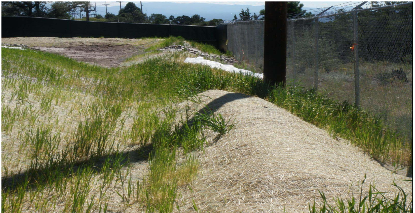
Photo 10551-1r.JPG (taken 09/20/10) L019A03010005 : Berms - Earthen Berm; L019A05020006 : Sediment Traps and Basins - Sediment Basin.
