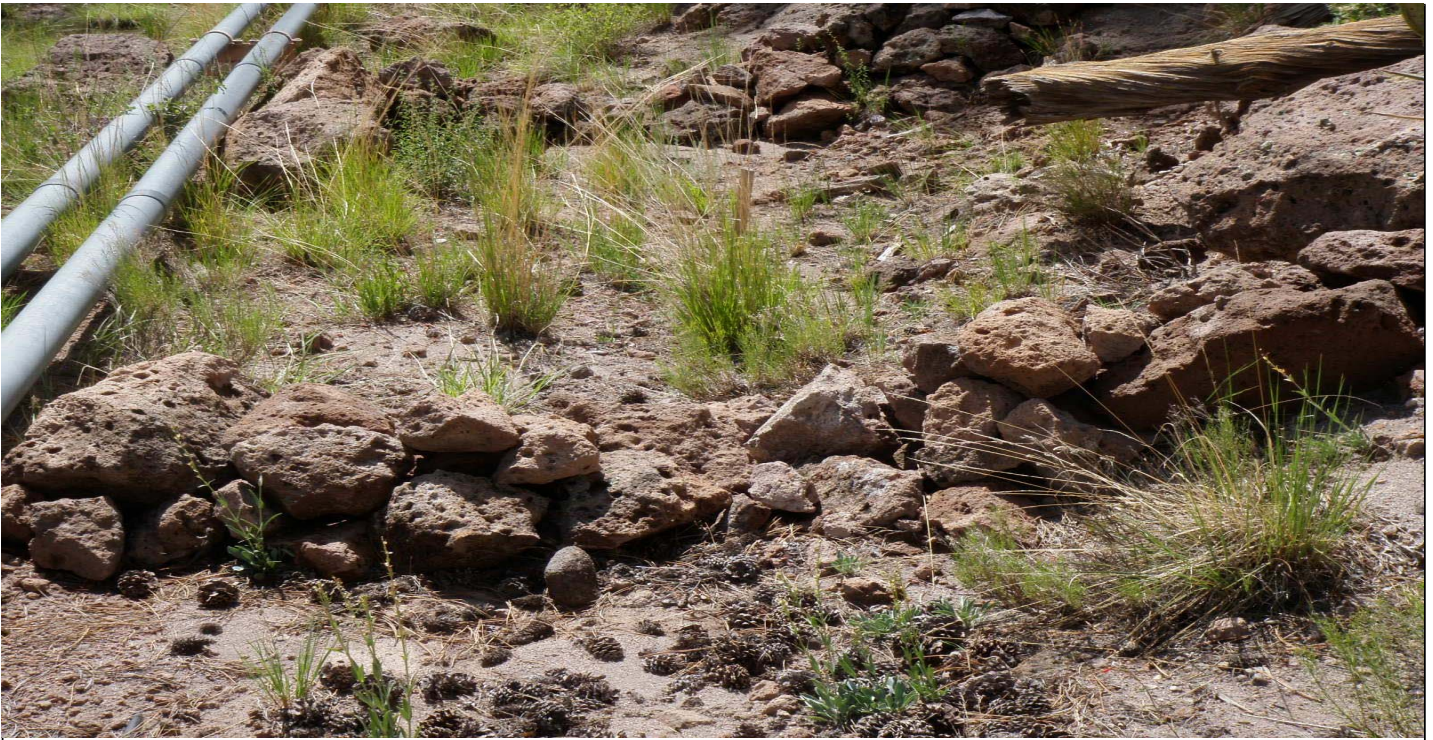
Photo 7449-2.JPG (taken 07/28/10) L01106010002 : Check Dam - Rock Check Dam; L01106010005 : Check Dam - Rock Check Dam.
