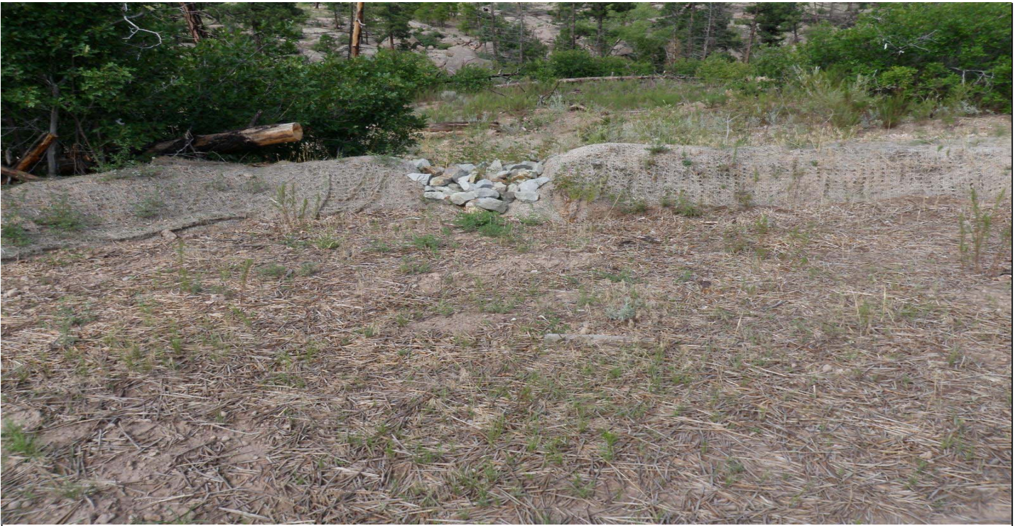
Photo 7482-1r.JPG (taken 08/10/10) C00601010008 : Seed and Mulch - Seed and Wood Mulch; C00601060007 : Seed and Mulch - Erosion Control Blanket; C00603010006 : Berms - Earthen Berm.
