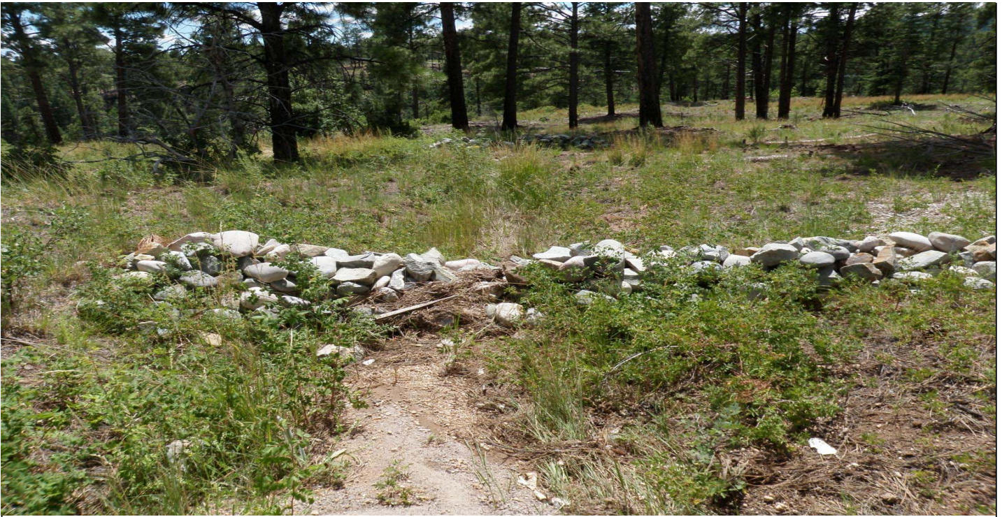
Photo 7506-1r.JPG (taken 08/11/10) J00506010008 : Check Dam - Rock Check Dam; J00506010009 : Check Dam - Rock Check Dam.
