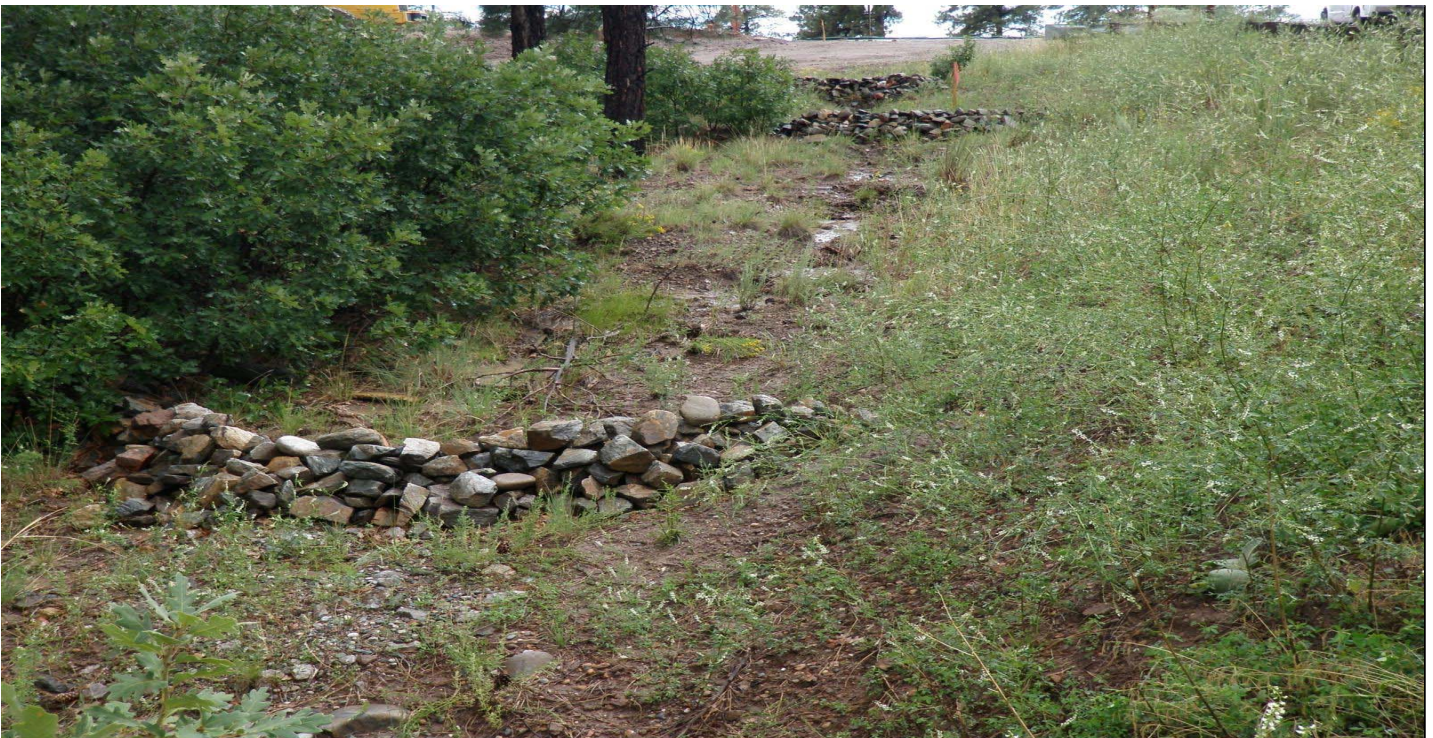
Photo 7489-1r.JPG (taken 08/09/10) M00606010010 : Check Dam - Rock Check Dam; M00606010011 : Check Dam - Rock Check Dam.
