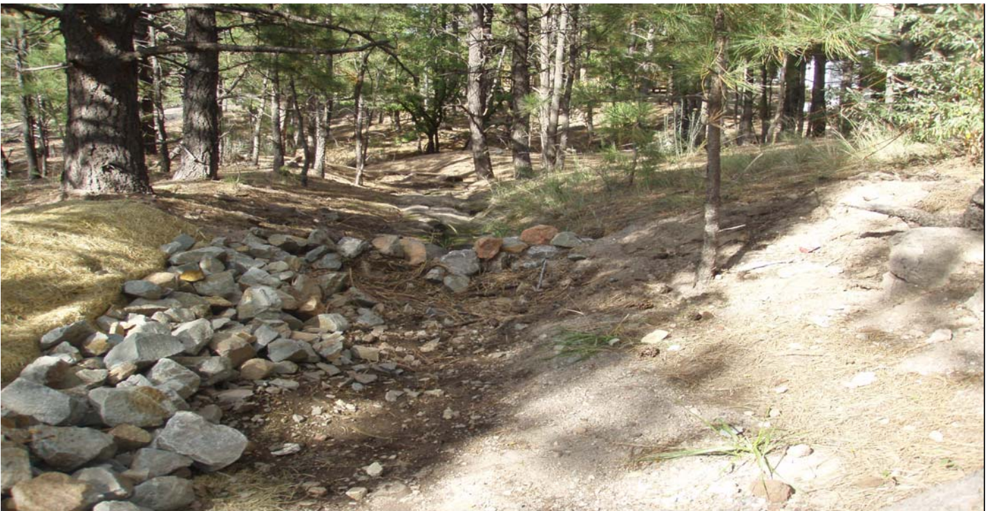
Photo 10870-2.JPG (taken 10/07/10) P00206010002 : Check Dam - Rock Check Dam.
