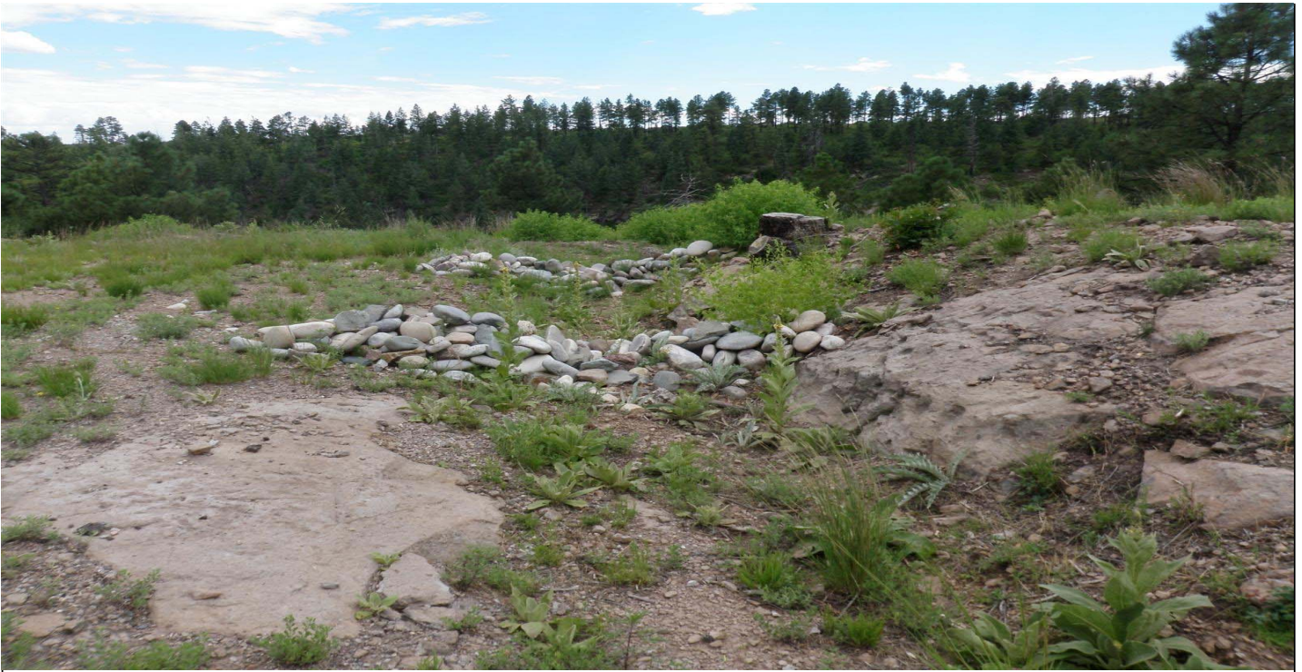
Photo 7511-1r.JPG (taken 08/12/10) J01006010008 : Check Dam - Rock Check Dam; J01006010009 : Check Dam - Rock Check Dam.
