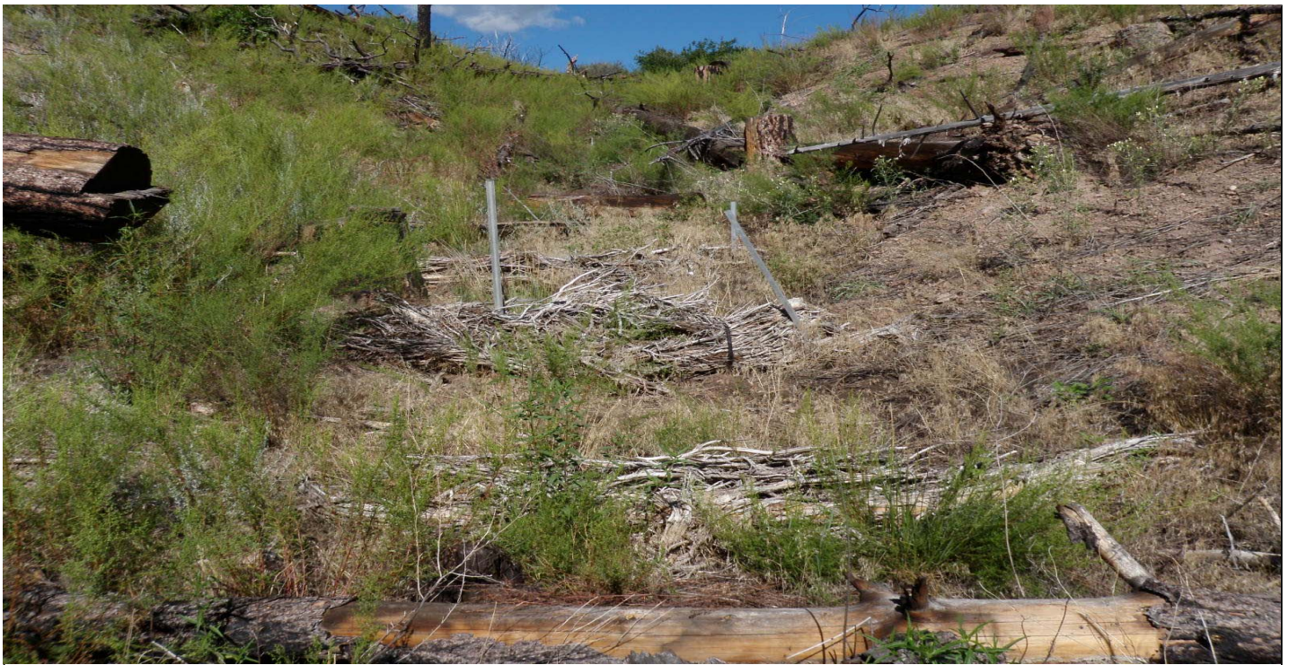
Photo 7444-1.JPG (taken 08/03/10) R00402020001 : Established Vegetation - Permanent Vegetation Forested/Needle Cast; R00406030002 : Check Dam - Juniper Bales; R00406030003 : Check Dam - Juniper Bales; R00406030004 : Check Dam - Juniper Bales.
