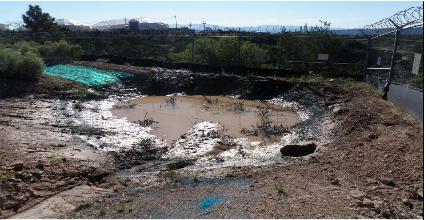
Photo 8504-3r.JPG (taken 08/20/10) J02605010005 : Sediment Traps and Basins - Sediment Trap.
