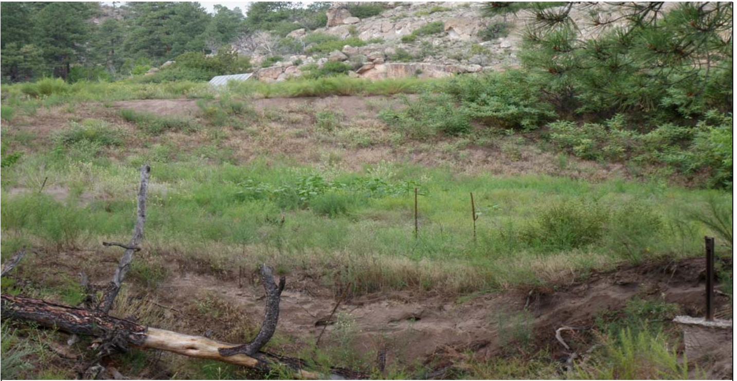
Photo 7471-2.JPG (taken 08/06/10) M02105010003 : Sediment Traps and Basins - Sediment Trap.
