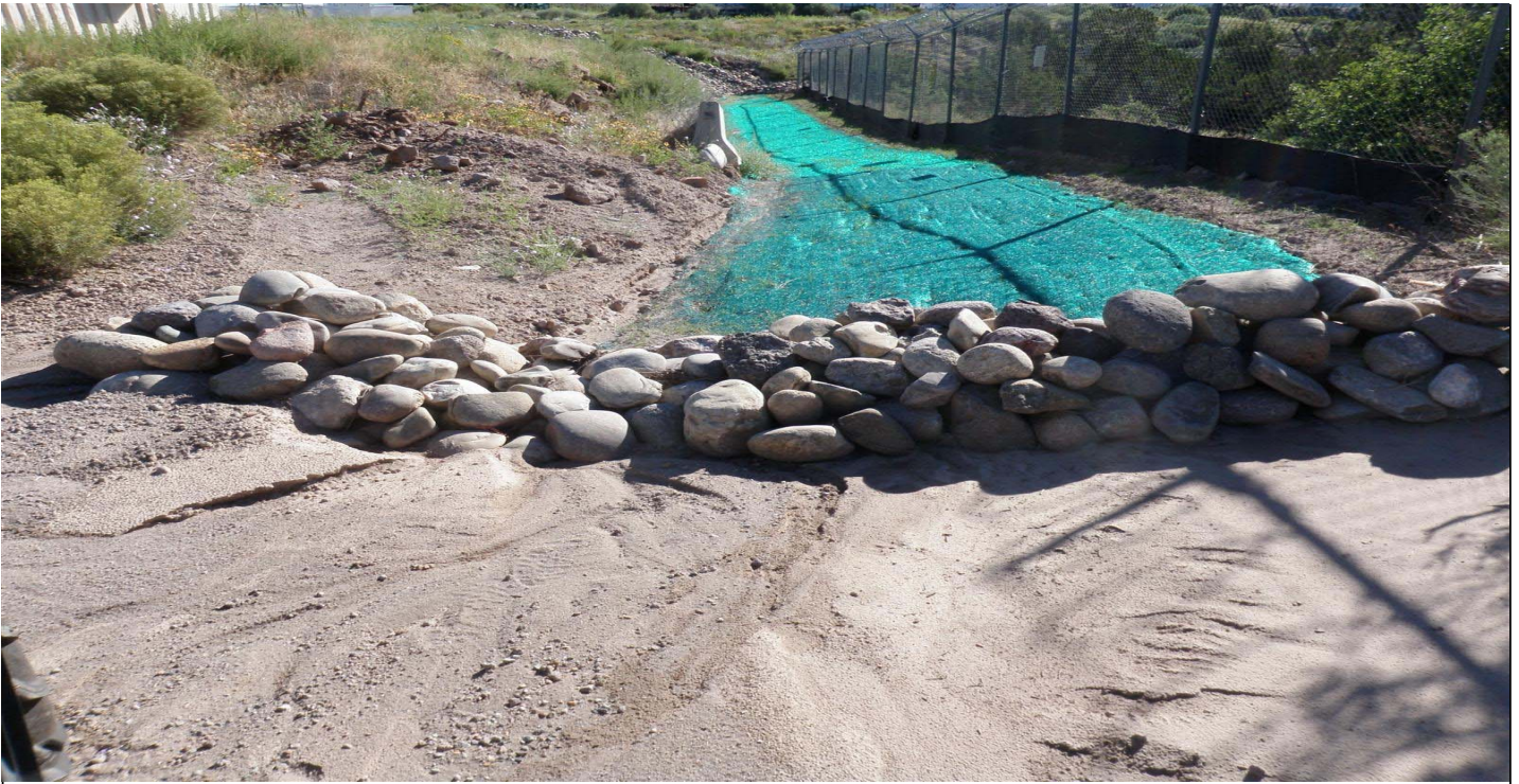
Photo 8504-1r.JPG (taken 08/20/10) J02601060002 : Seed and Mulch - Erosion Control Blanket; J02602010001 : Established Vegetation - Permanent Vegetation Grasses and Shrubs; J02606010006 : Check Dam - Rock Check Dam.
