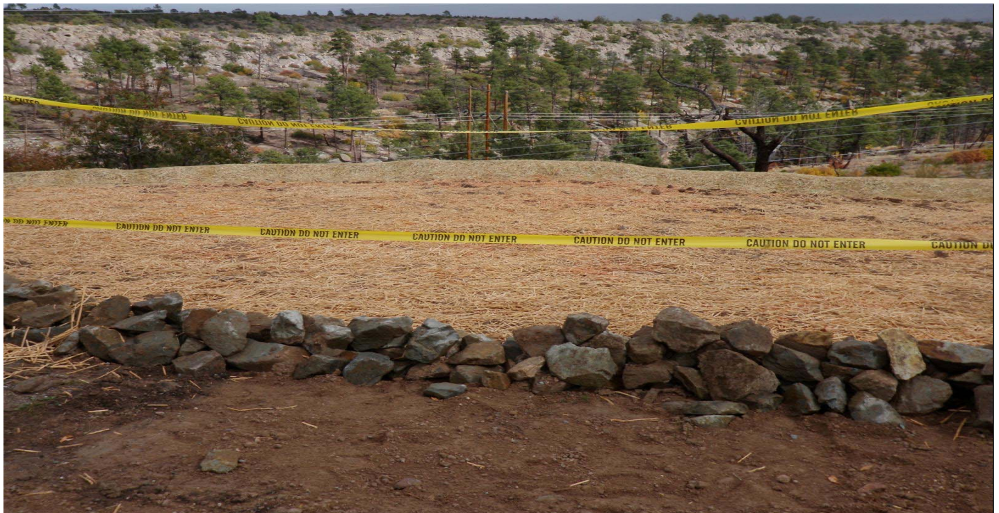
Photo 11462-1r.JPG (taken 10/22/10) C00801010011 : Seed and Mulch - Seed and Wood Mulch; C00803010010 : Berms - Earthen Berm; C00803120009 : Berms - Rock Berm.
