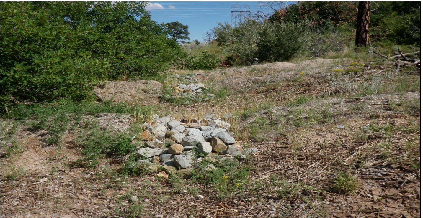
Photo 7481-4r.JPG (taken 08/10/10) C00701010013 : Seed and Mulch - Seed and Wood Mulch; C00701060010 : Seed and Mulch - Erosion Control Blanket; C00701060011 : Seed and Mulch - Erosion Control Blanket; C00701060012 : Seed and Mulch - Erosion Control Blanket; C00703010007 : Berms - Earthen Berm; C00703010008 : Berms - Earthen Berm; C00703010009 : Berms - Earthen Berm.
