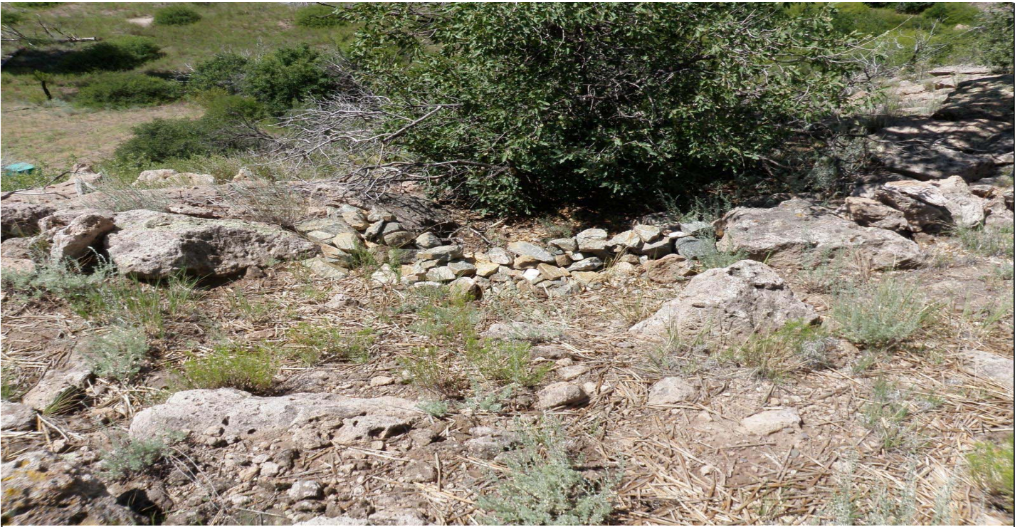
Photo 7486-3r.JPG (taken 08/10/10) M01606010008 : Check Dam - Rock Check Dam.
