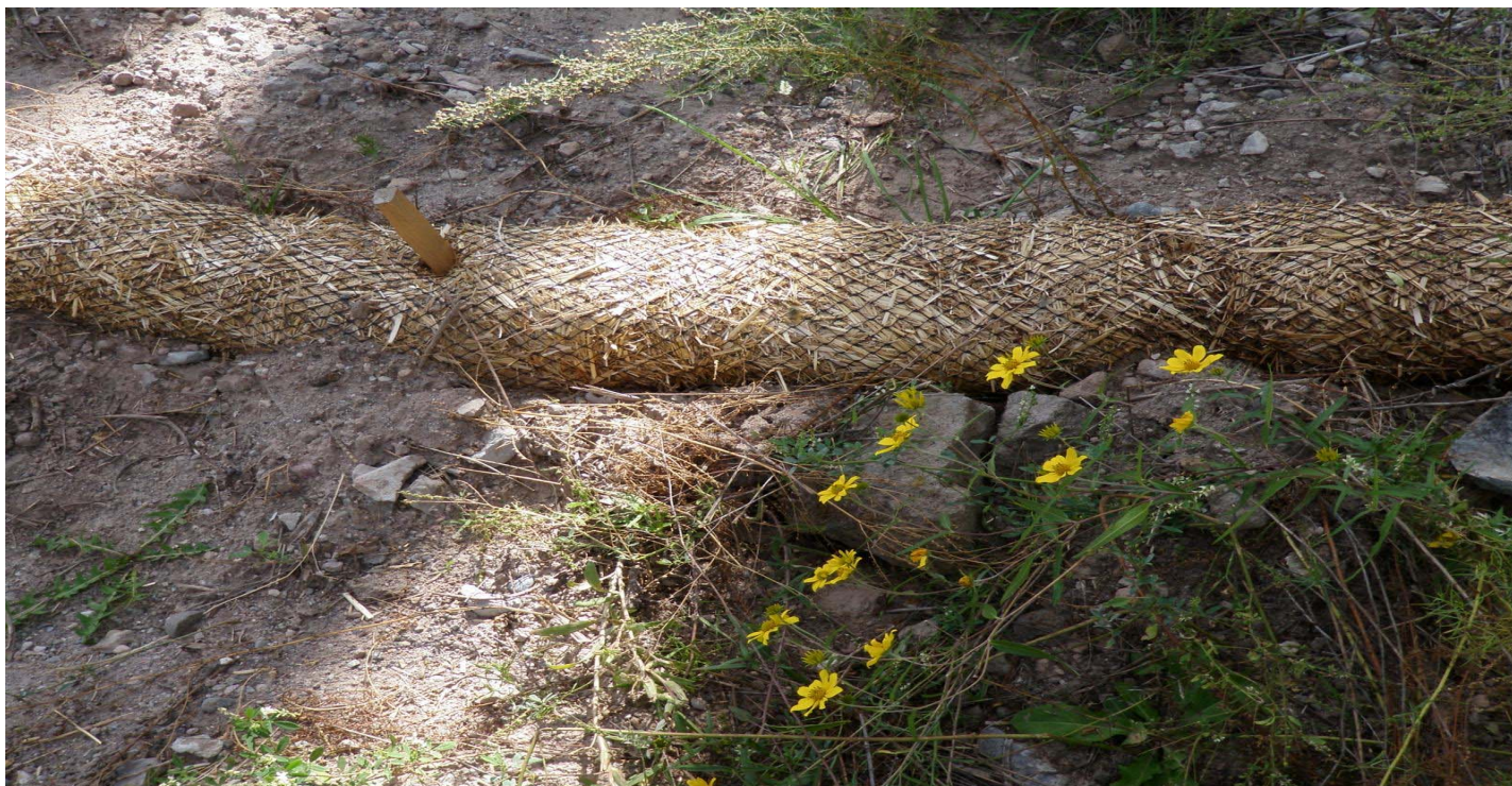
Photo 10562-1r.JPG (taken 09/14/10) L00203060009 : Berms - Straw Wattles.
