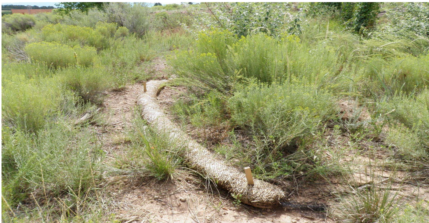
Photo 7491-2r.JPG (taken 08/09/10) S005A03060003 : Berms - Straw Wattles.
