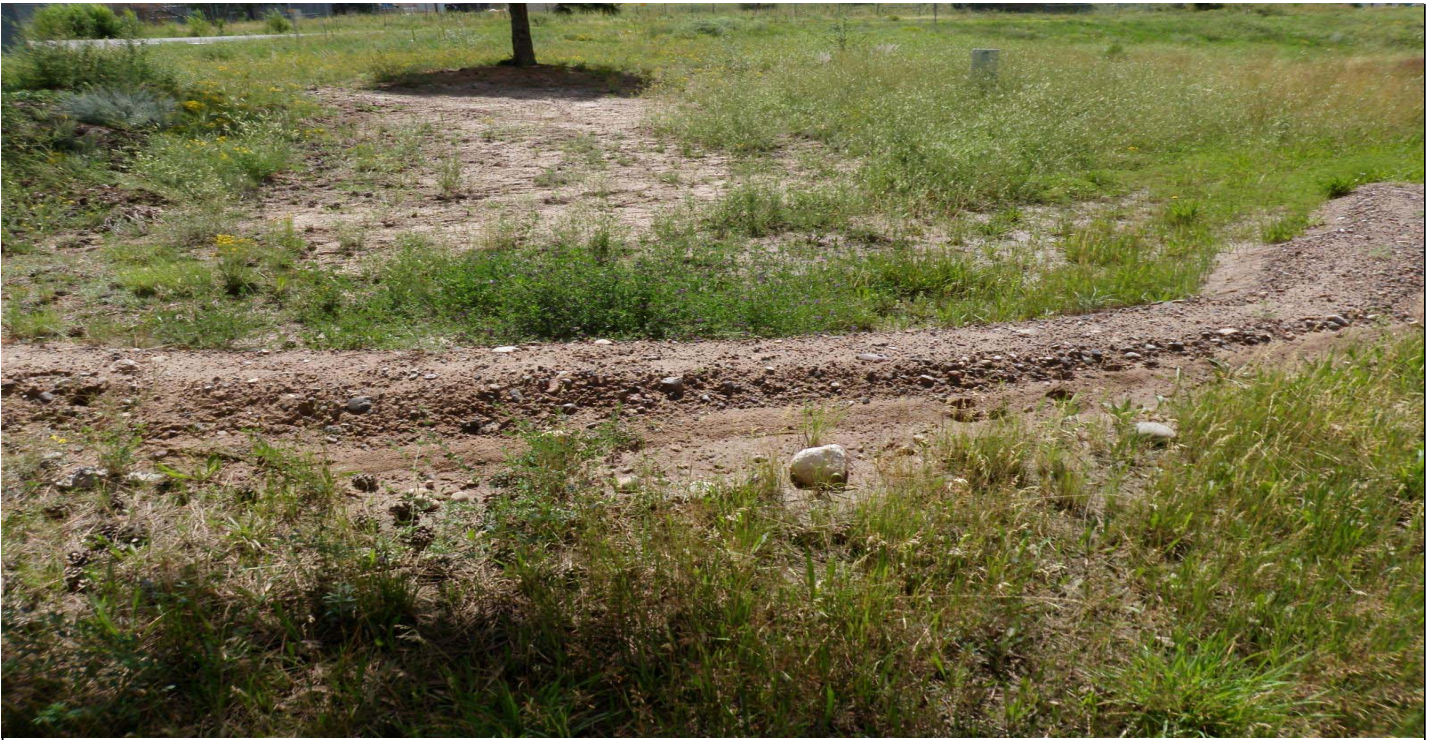
Photo 8501-1r.JPG (taken 08/19/10) S00503020006 : Berms - Base Course Berm.
