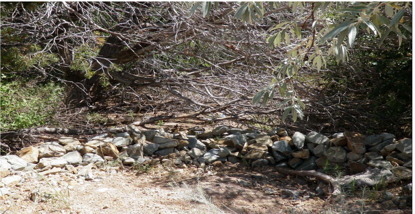
Photo 7416-3.JPG (taken 07/29/10) D00802020004 : Established Vegetation - Permanent Vegetation Forested/Needle Cast; D00806010005 : Check Dam - Rock Check Dam.
