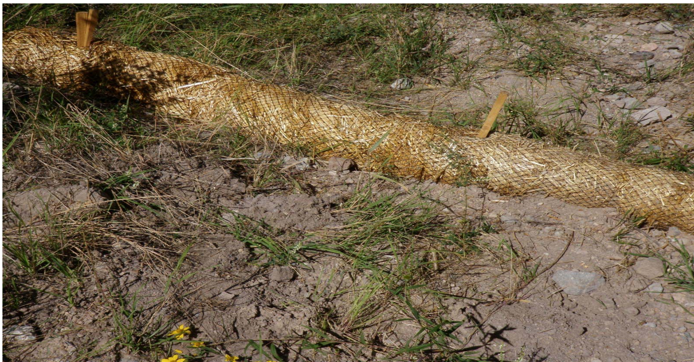
Photo 10562-3r.JPG (taken 09/14/10) L00203060011 : Berms - Straw Wattles.
