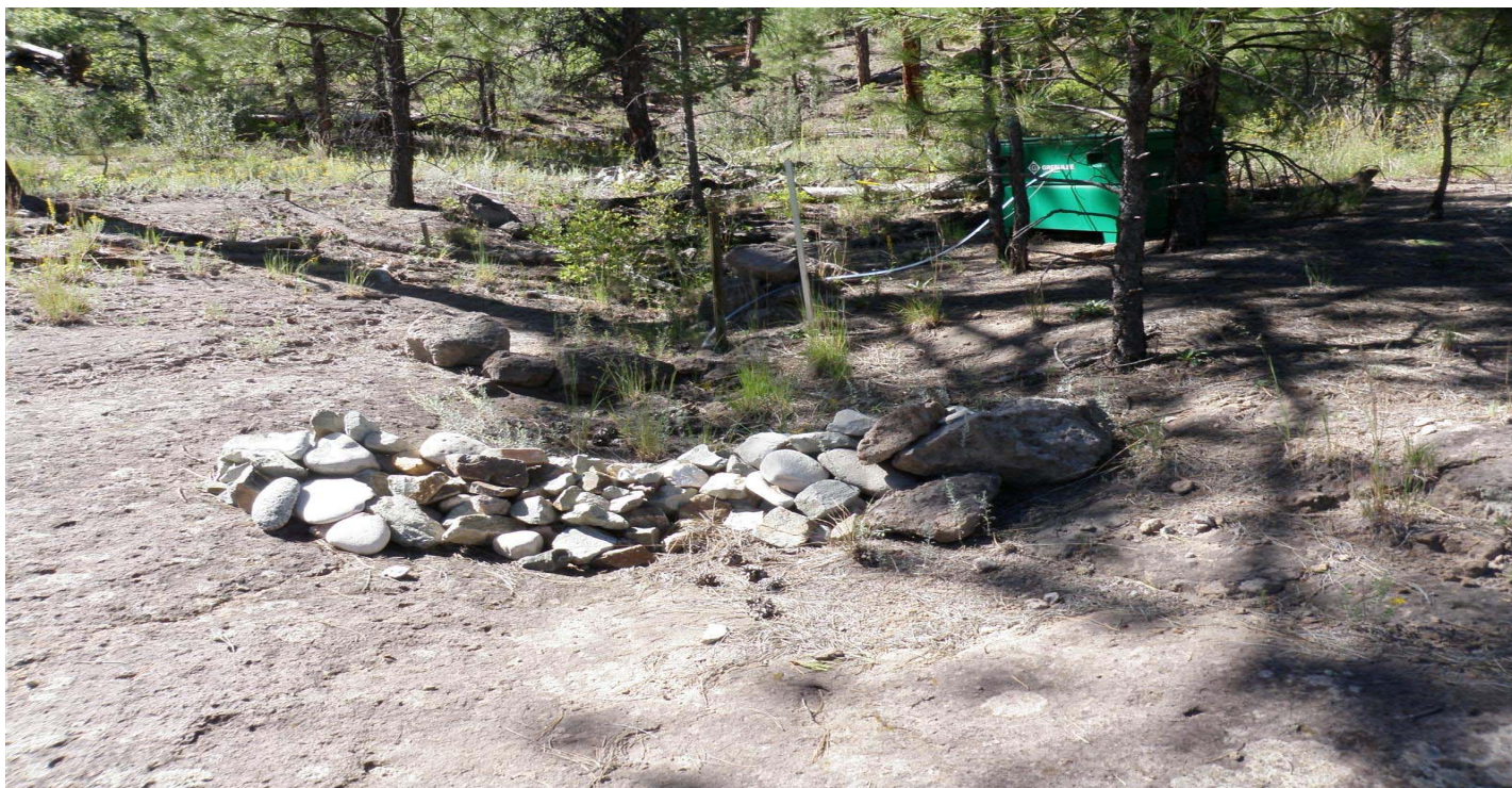
Photo 8665-1r.JPG (taken 09/02/10) T00906010007 : Check Dam - Rock Check Dam.
