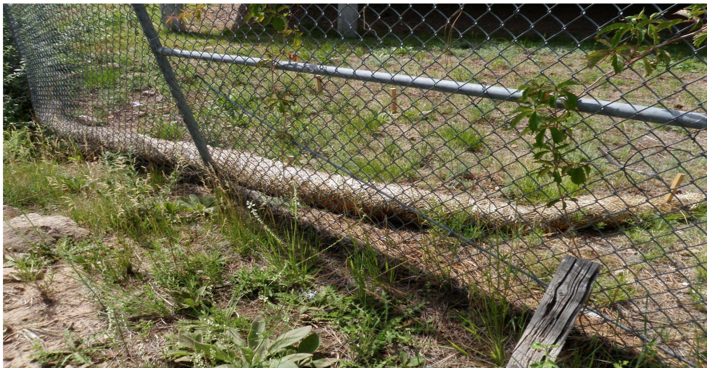
Photo 7491-1r.JPG (taken 08/09/10) S005A03060002 : Berms - Straw Wattles.
