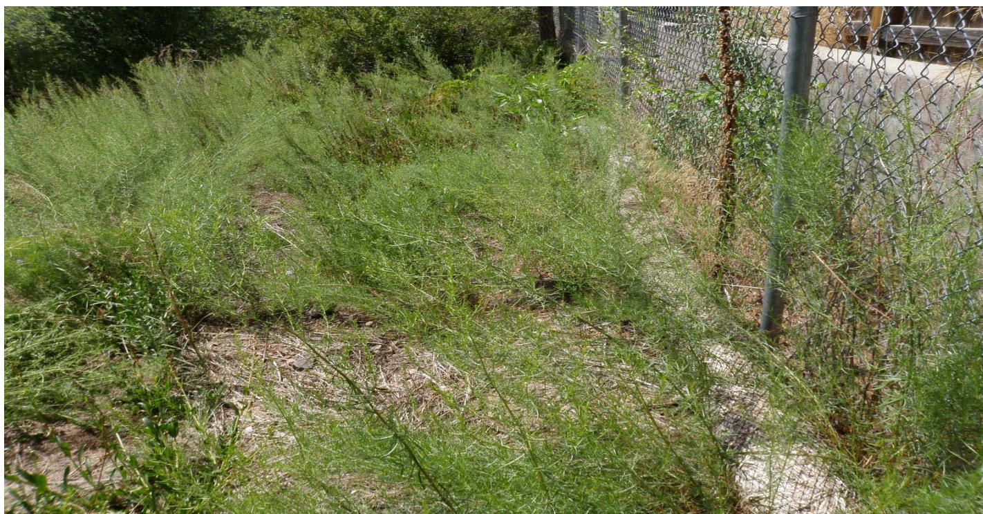
Photo 7421-1.JPG (taken 07/28/10) L00702010001 : Established Vegetation - Permanent Vegetation Grasses and Shrubs; L00703060003 : Berms - Straw Wattles; L00703080002 : Berms - Retaining Wall.
