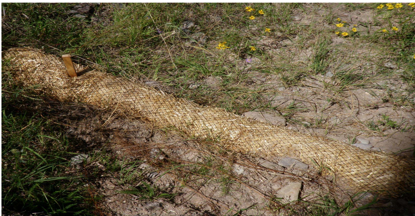
Photo 10562-2r.JPG (taken 09/14/10) L00203060008 : Berms - Straw Wattles.
