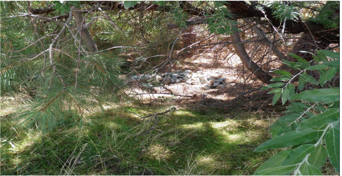
Photo 7469-2.JPG (taken 08/06/10) T00402010003 : Established Vegetation - Permanent Vegetation Grasses and Shrubs; T00402020002 : Established Vegetation - Permanent Vegetation Forested/Needle Cast; T00406010005 : Check Dam - Rock Check Dam.
