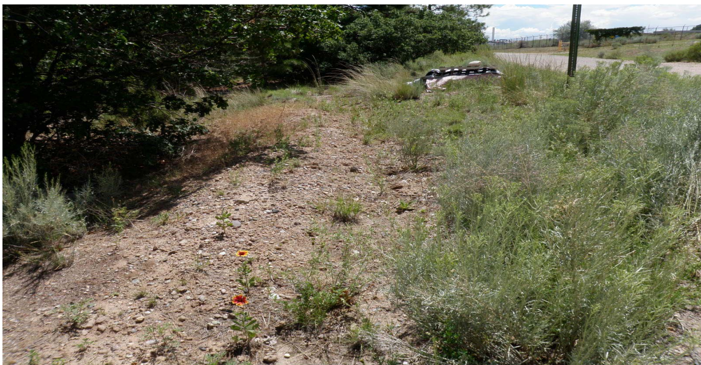
Photo 8656-6.JPG (taken 07/29/10) D00403010002 : Berms - Earthen Berm.
