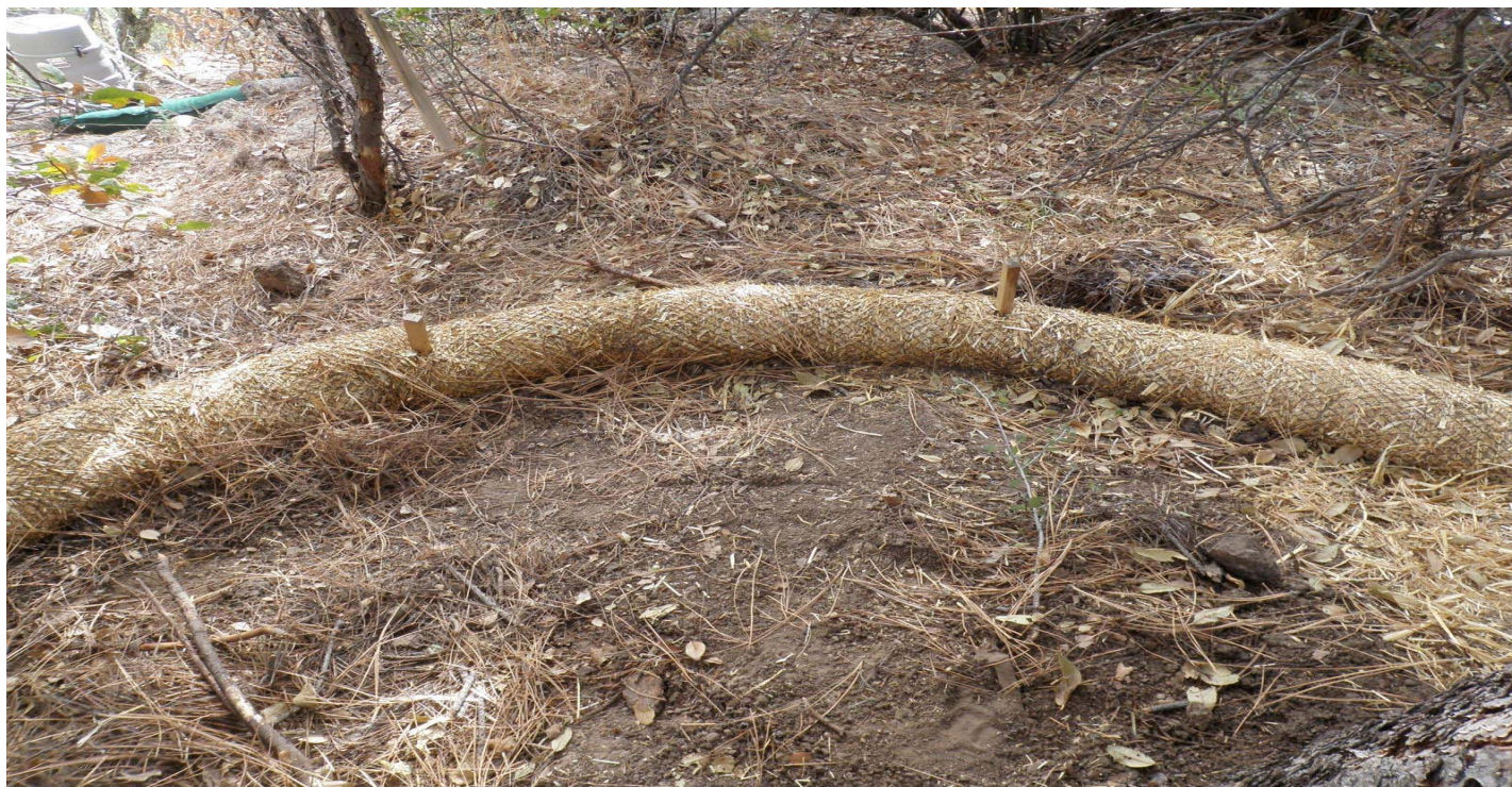
Photo 11700-1r.JPG (taken 11/15/10) L01603060008 : Berms - Straw Wattles.
