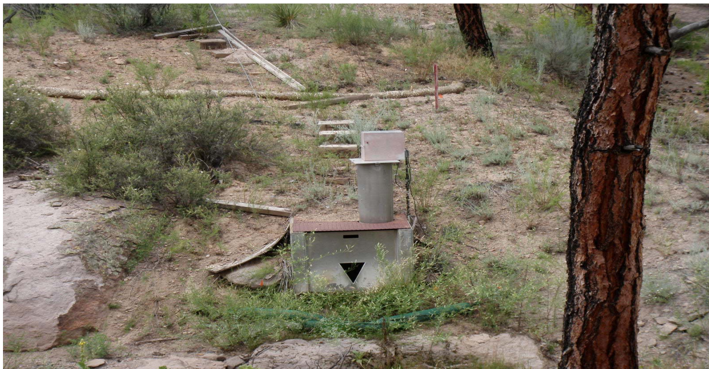
Photo 7455-1.JPG (taken 08/04/10) T00803060002 : Berms - Straw Wattles; T00803100003 : Berms - Gravel Bags.
