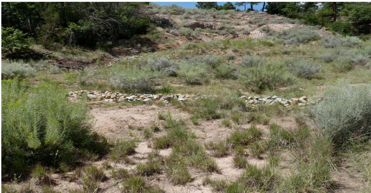
Photo 8656-5.JPG (taken 07/29/10) D00403120009 : Berms - Rock Berm.
