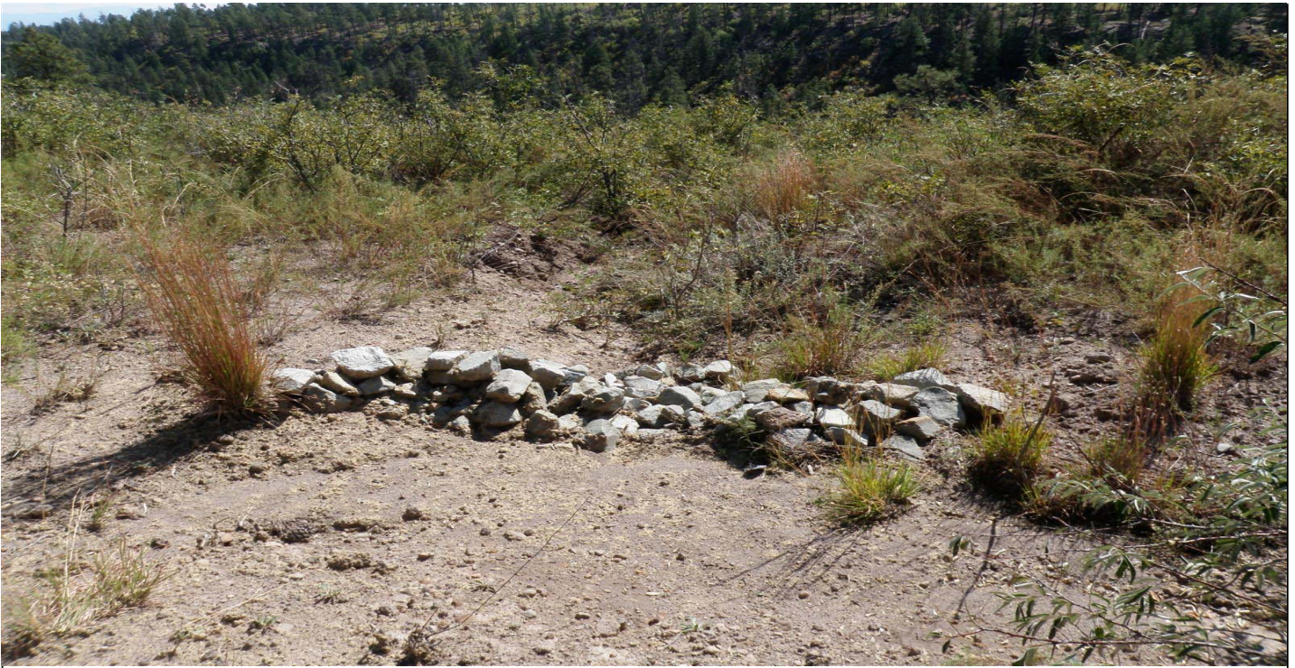
Photo 10864-7r.JPG (taken 10/07/10) J01302010002 : Established Vegetation - Permanent Vegetation Grasses and Shrubs; J01306010008 : Check Dam - Rock Check Dam.
