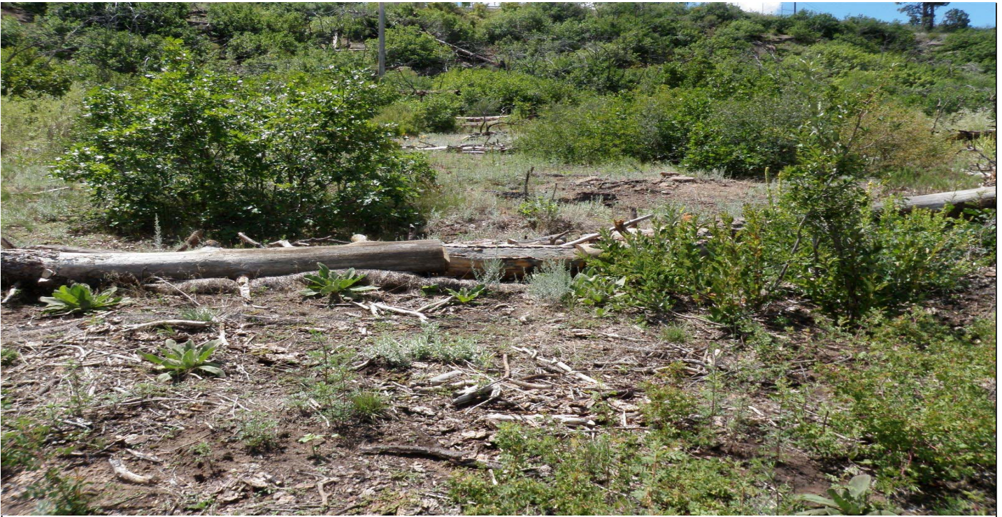
Photo 8503-5r.JPG (taken 08/19/10) C00306020014 : Check Dam - Log Check Dam.
