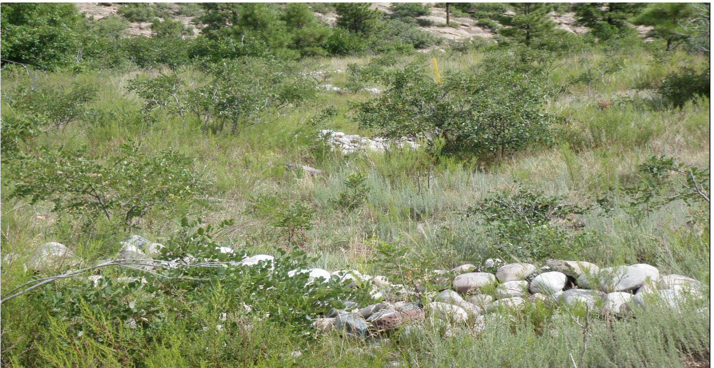
Photo 8516-2.JPG (taken 08/04/10) W02002010003 : Established Vegetation - Permanent Vegetation Grasses and Shrubs; W02006010001 : Check Dam - Rock Check Dam.
