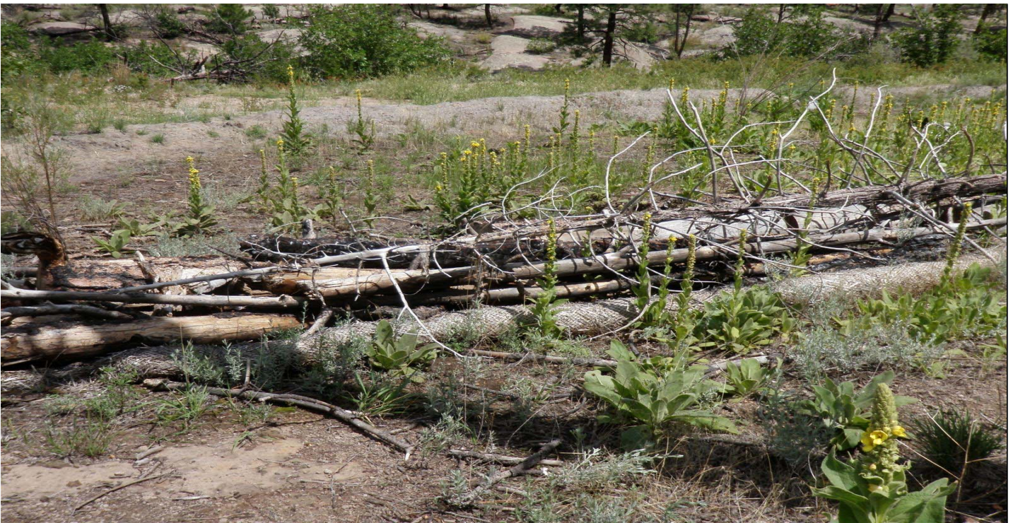
Photo 8503-6r.JPG (taken 08/19/10) C00302010008 : Established Vegetation - Permanent Vegetation Grasses and Shrubs; C00303010011 : Berms - Earthen Berm; C00306020012 : Check Dam - Log Check Dam.
