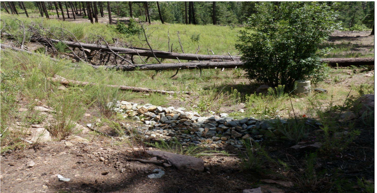
Photo 7507-3r.JPG (taken 08/11/10) J00602010001 : Established Vegetation - Permanent Vegetation Grasses and Shrubs; J00606010007 : Check Dam - Rock Check Dam.
