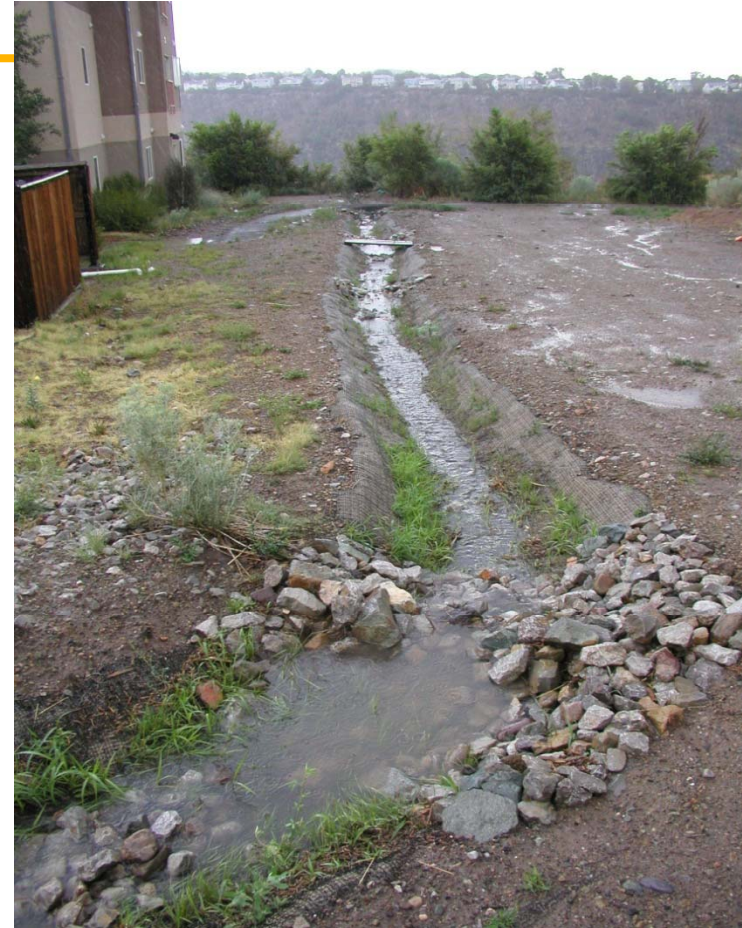
Storm water run-on from private land owners
