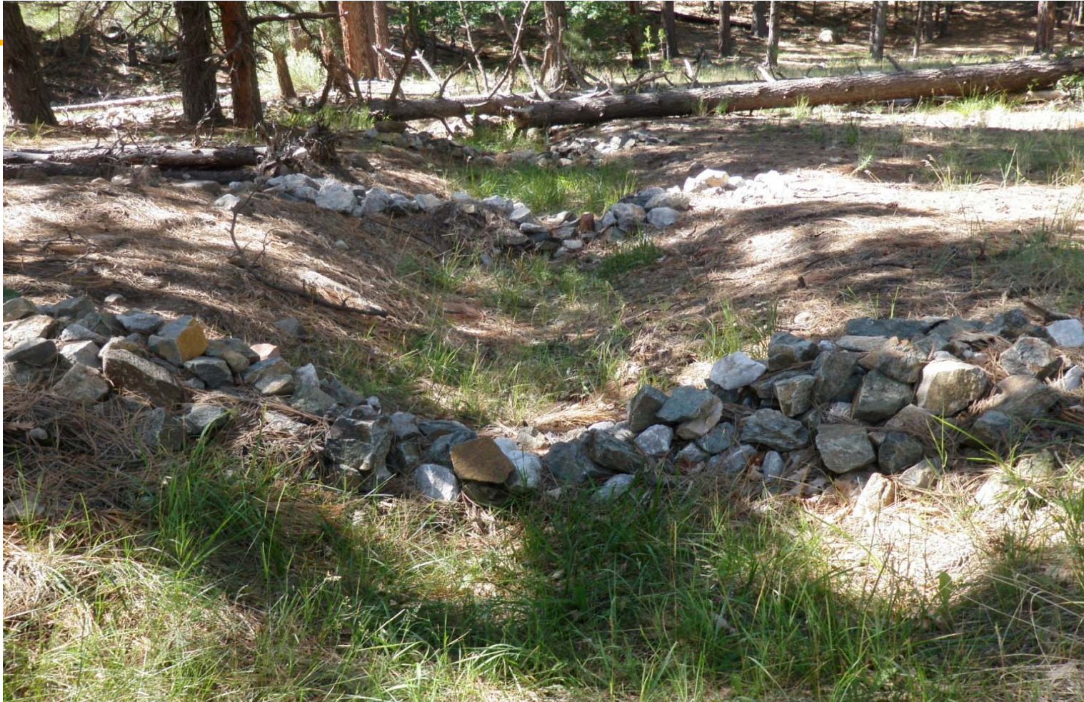
Rock check dams installed in former outfall drainage to assist with site stabilization.
