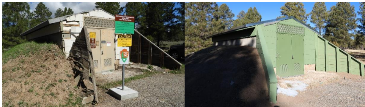
Figure 3-1. The Technical Area 16 Manhattan Project magazine in a state of disrepair before preservation work (left) and after preservation work was completed (right). The Laboratory's preservation work means that the magazine should stand for many more years.
