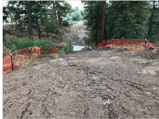
Figure 3-1: Erosion at SWMU-03-010(a)
