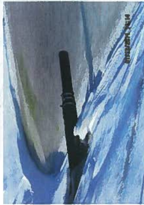
East basin influent pipe ( 1-13-2011 )
