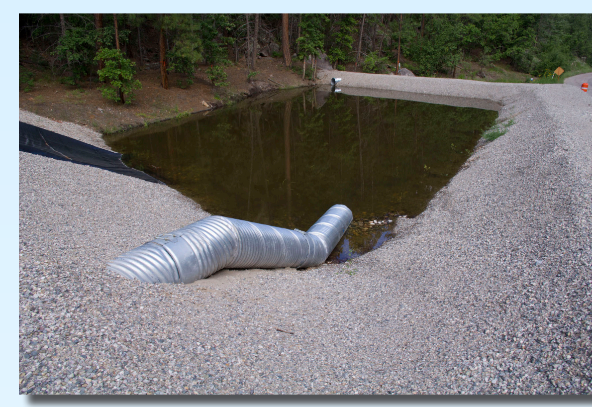
The retention basin in upper Los Alamos Canyon traps and settles sediment while allowing continued flow of storm water.
