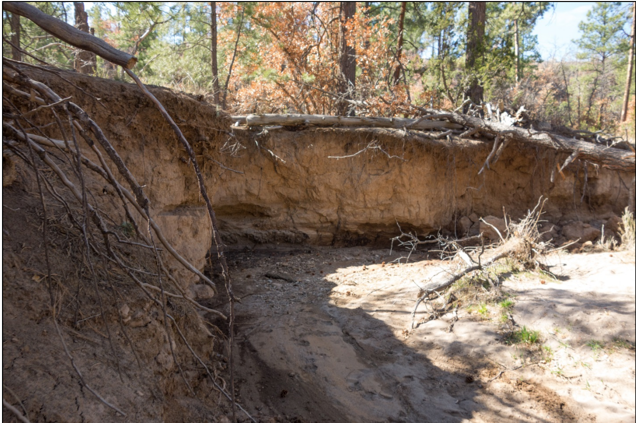
Photograph 3. Severe bank undercutting.
